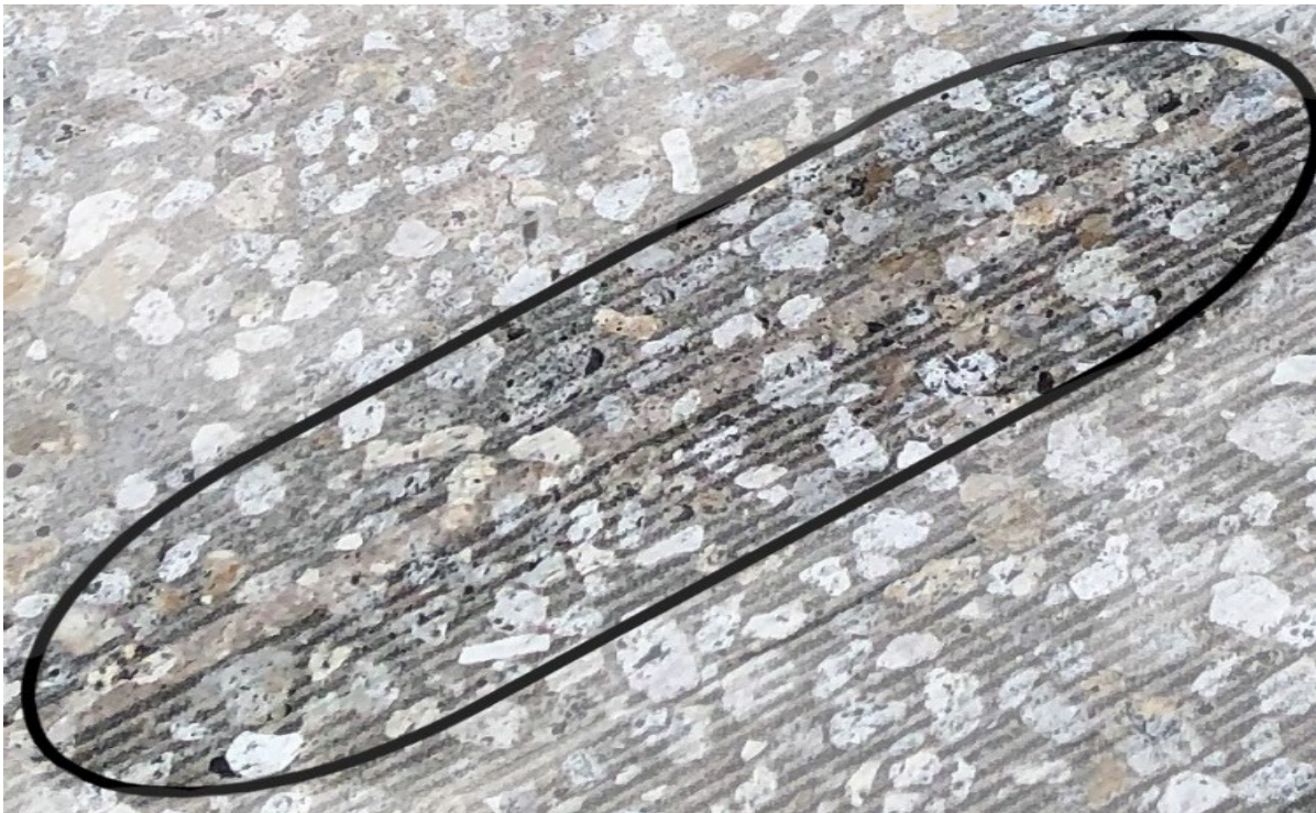
Figure 5-22. Texture feature in left-hand wheel path at SR-600 EB location.
