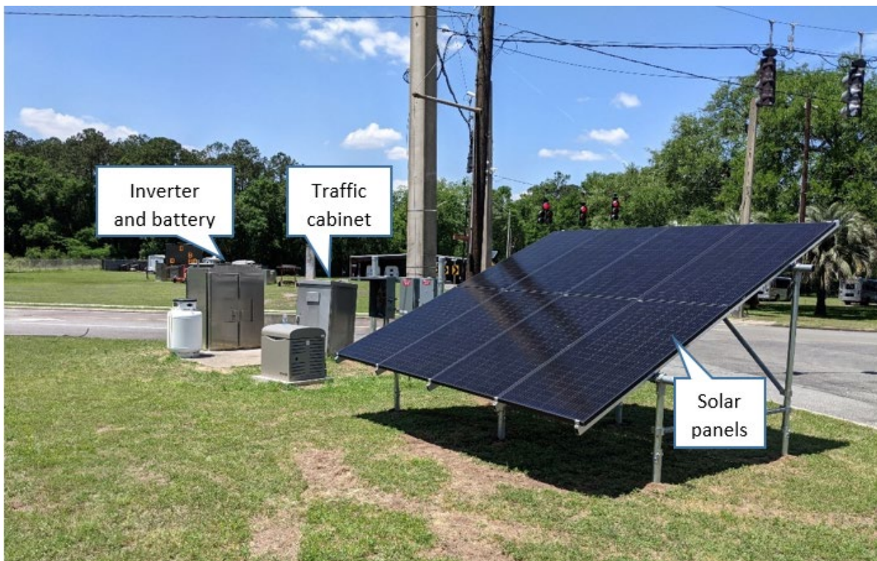
Figure 54. Battery + solar system at test site
