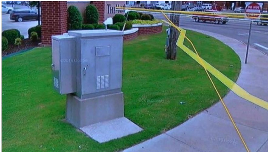
Figure 3. Battery backup system for traffic signal in Jonesboro, AR
