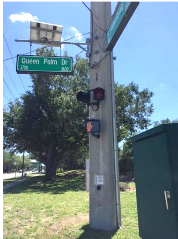
Figure 16. Solar-powered signal system in Hillsborough County, FL
