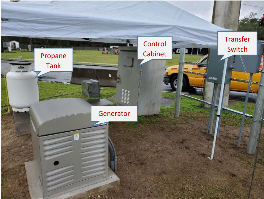
Figure 44. Propane generator backup power supply system at test site
