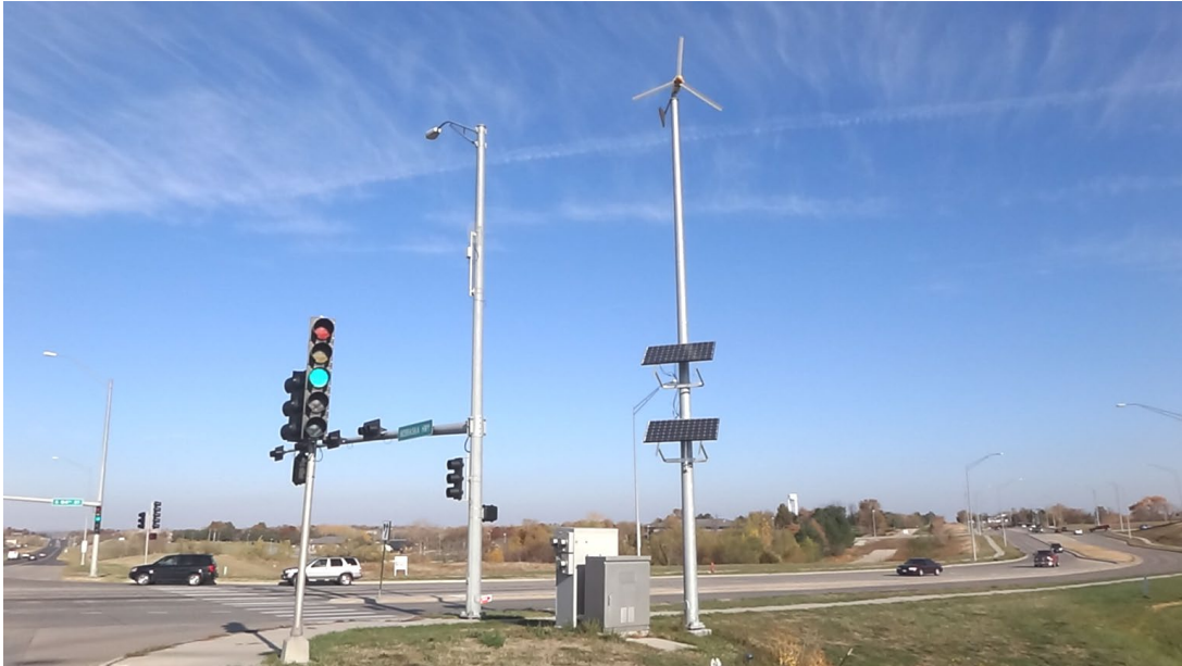
Figure 21. Test site in Lincoln, NE—one 1.0-kW wind turbine, two 210-W PV panels, four 6-V 305-Ah lead-acid batteries
