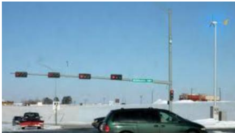
Figure 19. Wind-powered traffic lights in Lincoln, NE
