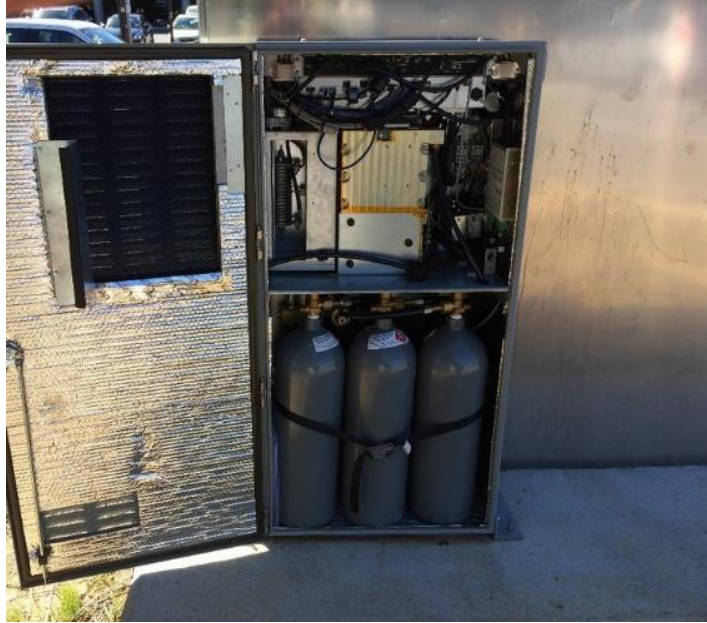
Figure 5. Intersection hydrogen fuel cell backup generator, Alexandria, VA
