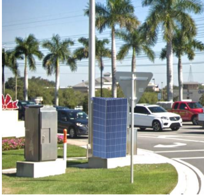
Figure 11. Solar panels mounted on top and sides of traffic signal cabinet
