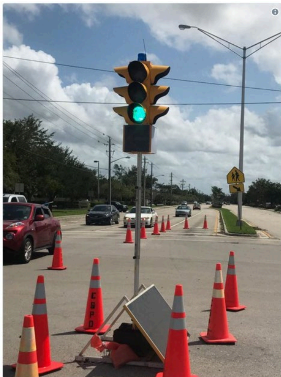
Figure 17. Temporary solar traffic signals in Coral Springs, FL
