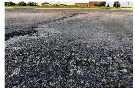
Open-graded friction courses can be subject to raveling, which leads to a rough pavement texture and further damage.
