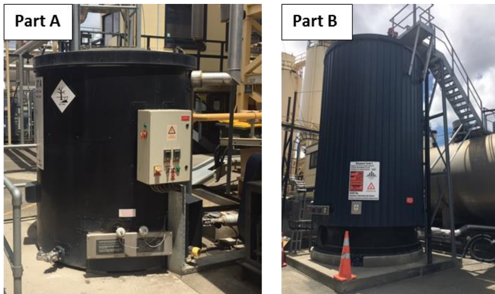
Figure 25. Introduction of Epoxy Asphalt Components at a Drum Plant in New Zealand (Van de Linda, 2019)
