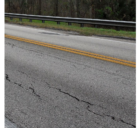
Moisture can cause set up pavement to lose asphalt and crack, leading to pavement loss.
