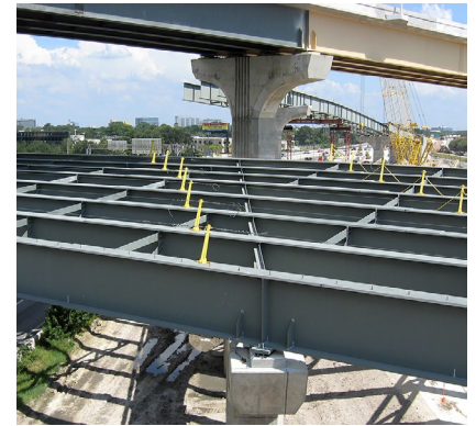
Continuous-span steel I-girder bridge with skewed support, Spruce Street Interchange, Tampa, Florida
