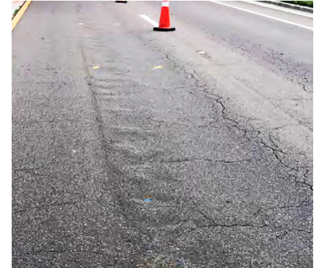
This pavement shows several kinds of distress: pavement blistering in the center; shoving and cracking right of center; and rutting far right.
