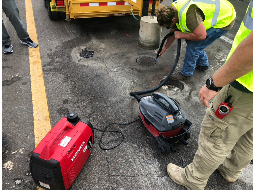
Figure 3-20. Partial-Depth Wet-Coring and Vacuuming of 12-in Diameter AC Samples Prior to Dry Coring
