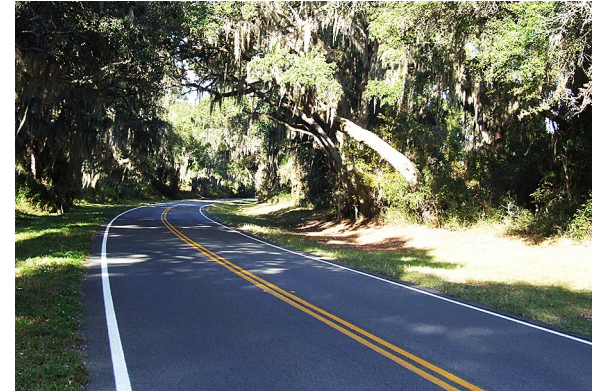
Low volume, rural roads are good candidates for paving with mixes containing high amounts of reclaimed asphalt pavement.
