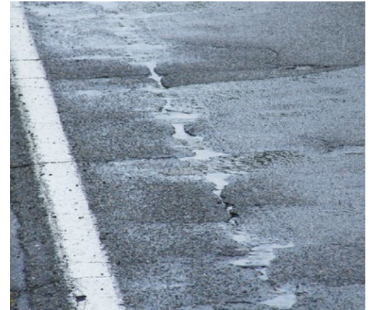
An inadequate joint between old and new asphalt on a widened road can become a site of deterioration requiring premature maintenance.
