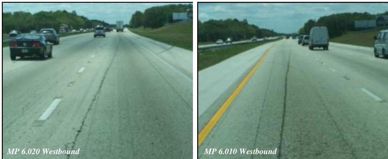
Figure 19. Diagonal reflective cracking in transition area of SR 400 widening.
