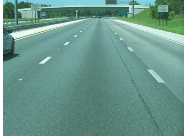
Longitudinal joint reflective cracking
