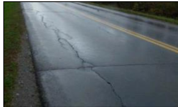
Widening roadways in poor condition
