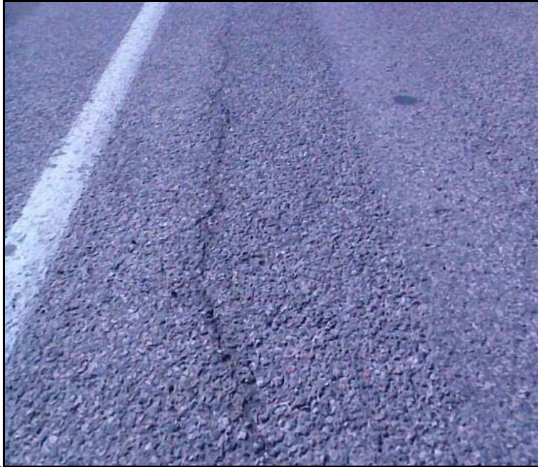
Figure 14. Typical longitudinal crack observed.
