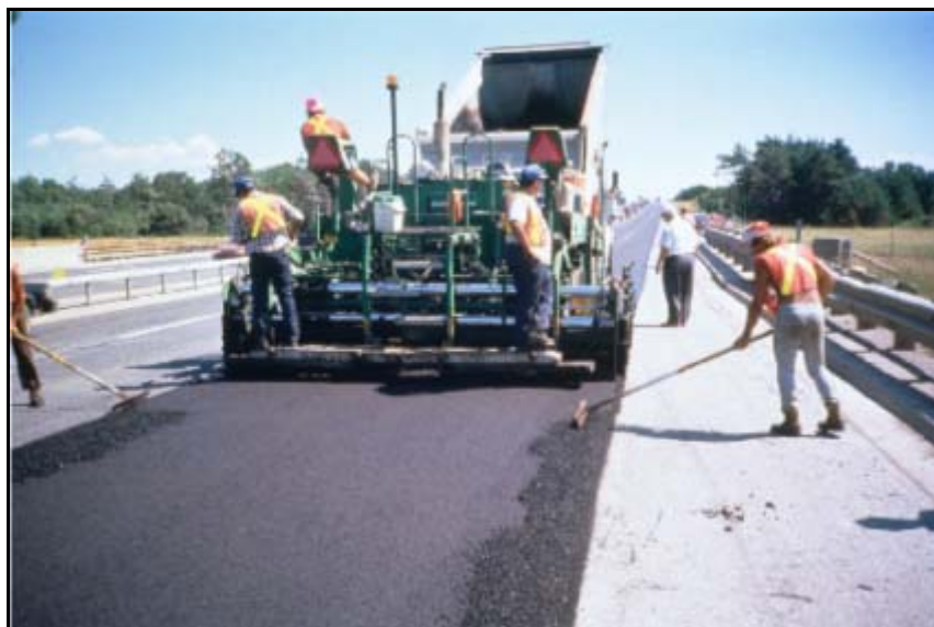
Figure 7. Improper raking of the longitudinal joint.
