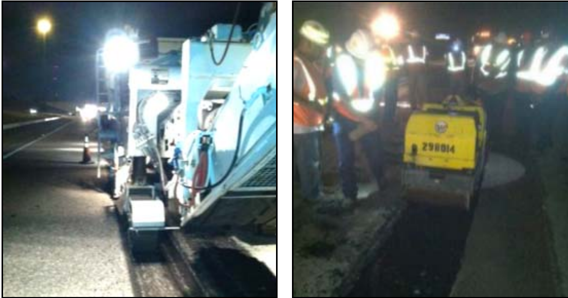
Figure 37. Milling and overlay of longitudinal crack.
