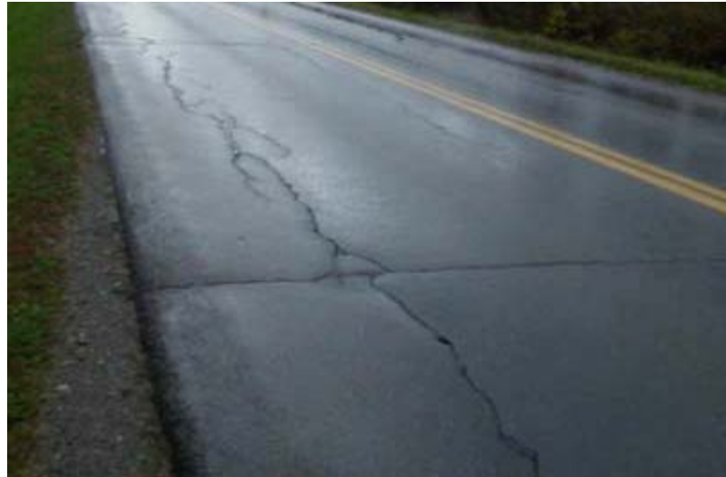
Flexible pavement section in poor condition.
