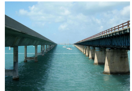
The piers of the Seven-Mile Bridge in the Florida Keys are constantly subjected to waves and currents.
