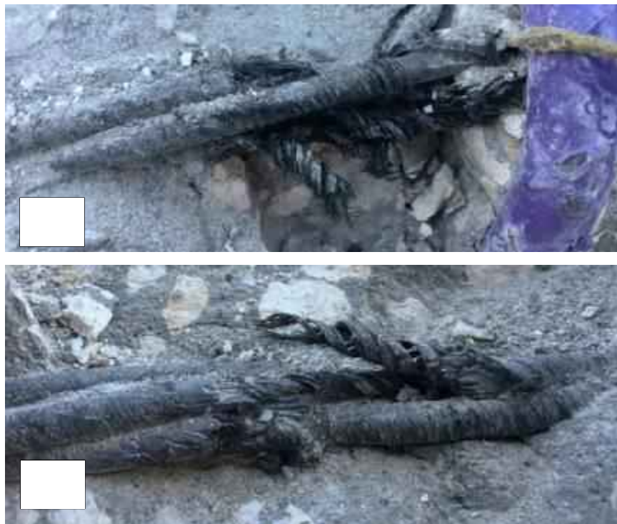
Figure 6.21: A close up view of the strand rupture after 3 months exposure (a) top beam (b) bottom beam.
