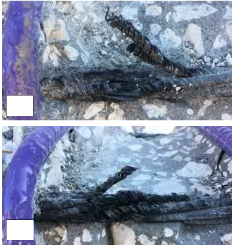
Figure 6.32: A close up view of the strand rupture after 18 months exposure (a) top beam (b) bottom beam.
