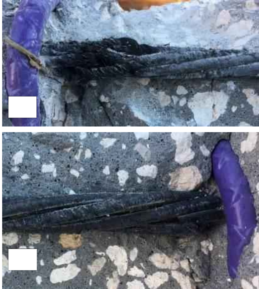
Figure 6.36: A close up view of the strand rupture after 18 months exposure to sustained load only (a) top beam (b) bottom beam.
