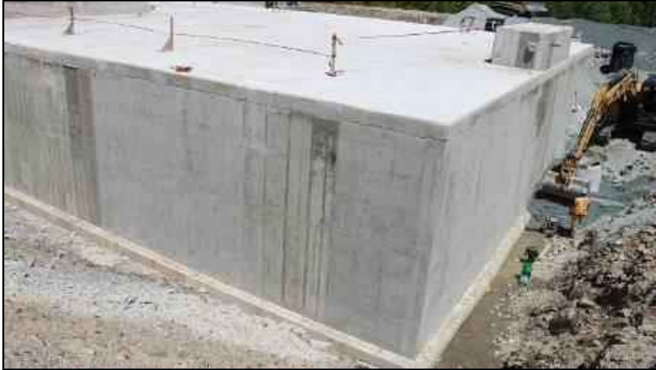
(b) Over view of the tank
