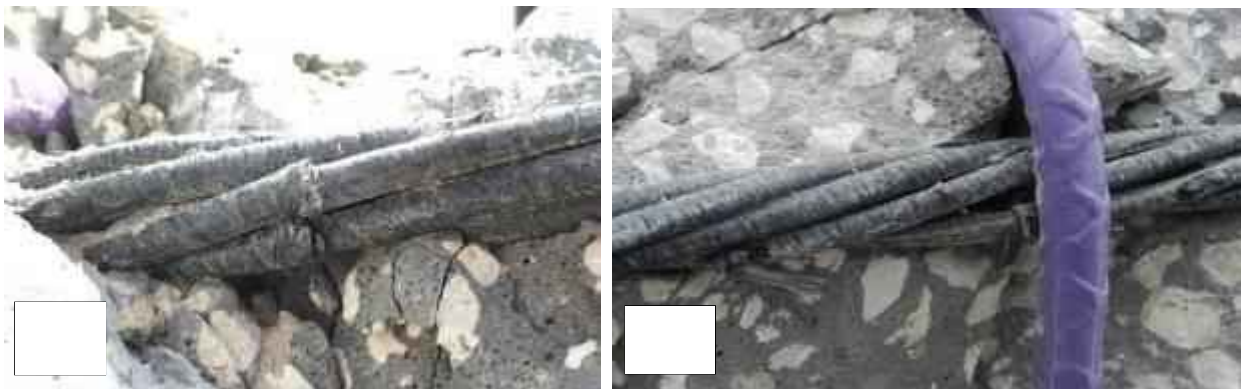
Figure 6.17: Rupture of strands (a) Control beam #1 (b) Control beam #2
