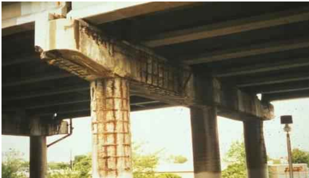
Figure 2.7: Concrete structure deteriorated by the corrosion of steel reinforcement-t
