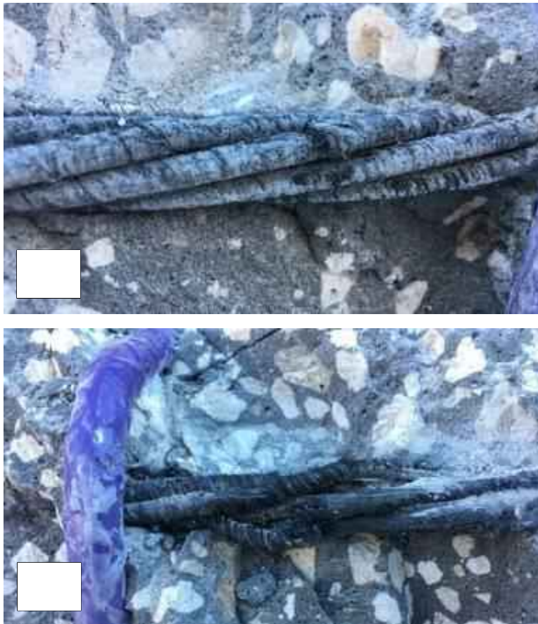
Figure 6.25: A close up view of the strand rupture after 6 months exposure (a) top beam (b) bottom beam.
