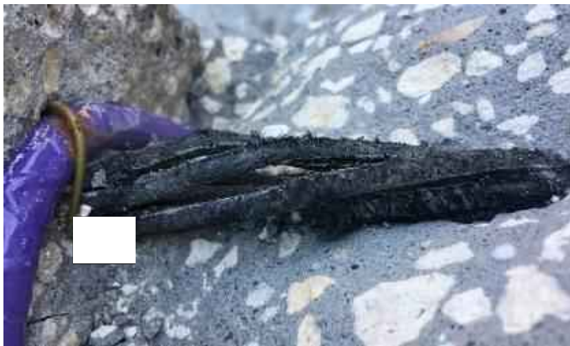
Figure 6.29: A close up view of the strand rupture after 12 months exposure (a) top beam (b) bottom beam
