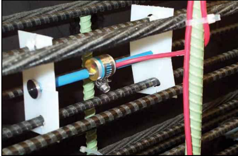
a) Leadline tendons and CFRP strands in reinforcement cage of double-T girders
