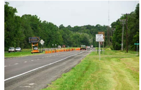
We drive by them every day without noticing, but properly maintained shoulders and ditches are critical to driver safety and roadway integrity.
