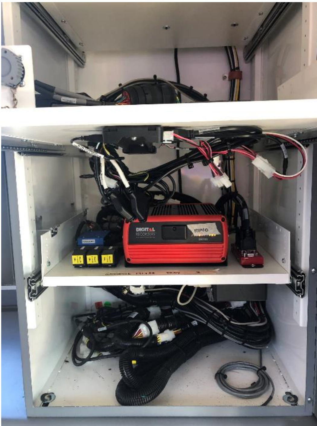
Figure D-7 – Junction box under shelf
