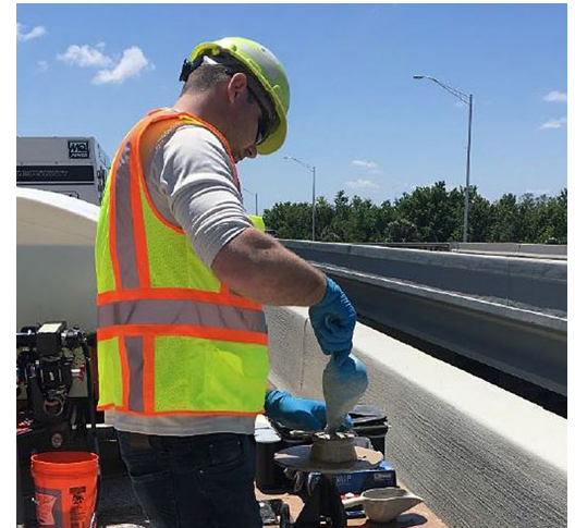
A worker conducts a slump test of freshly made UHPC. This simple test helps verify the consistency of a batch of concrete.
