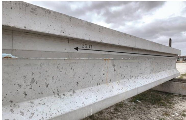
Figure 5.18 Formation of crack on specimen SS-2 at a distance of 20 ft from west end (north side)
