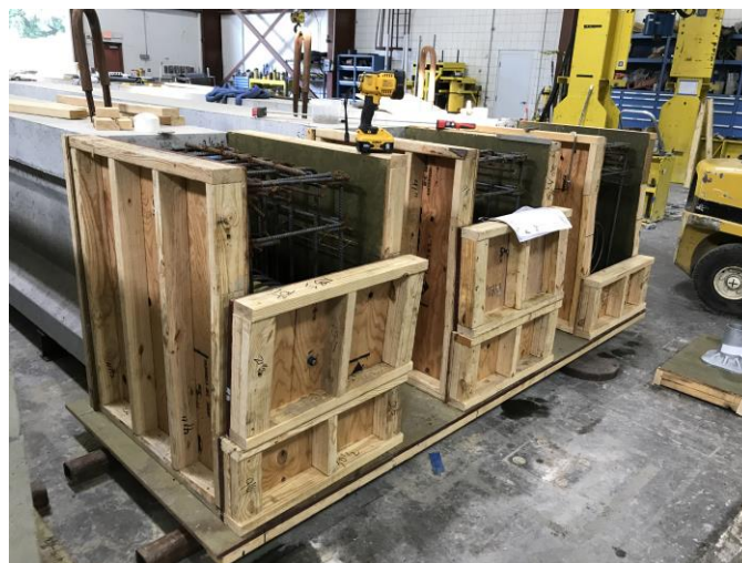
Figure 5.20 Installation of formwork for fabrication of end blocks for precast SS specimens
