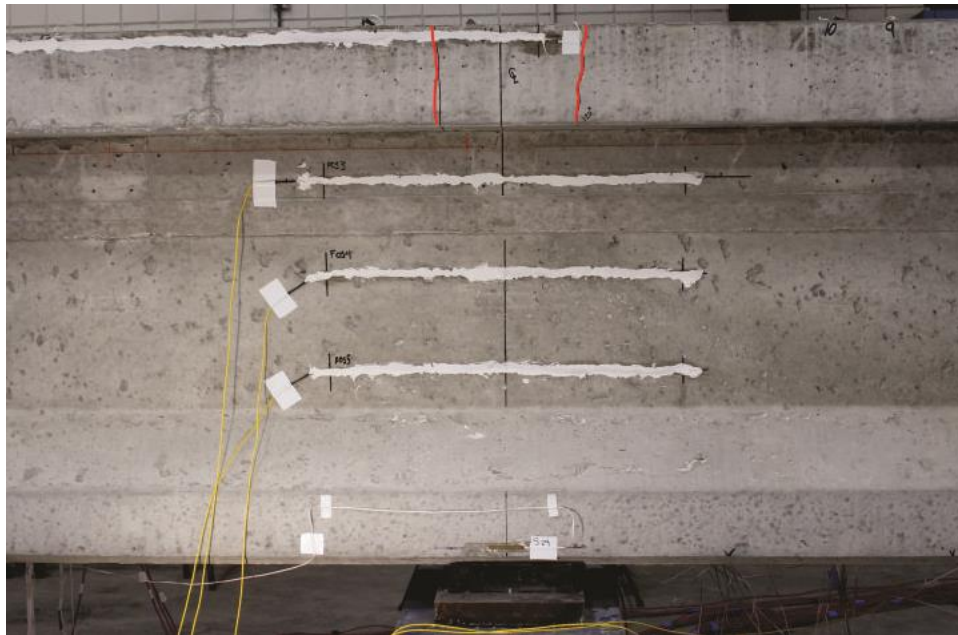
Figure E.8 Specimen NB-1: first observed cracks (marked in red) at P = 120 kip on east side
