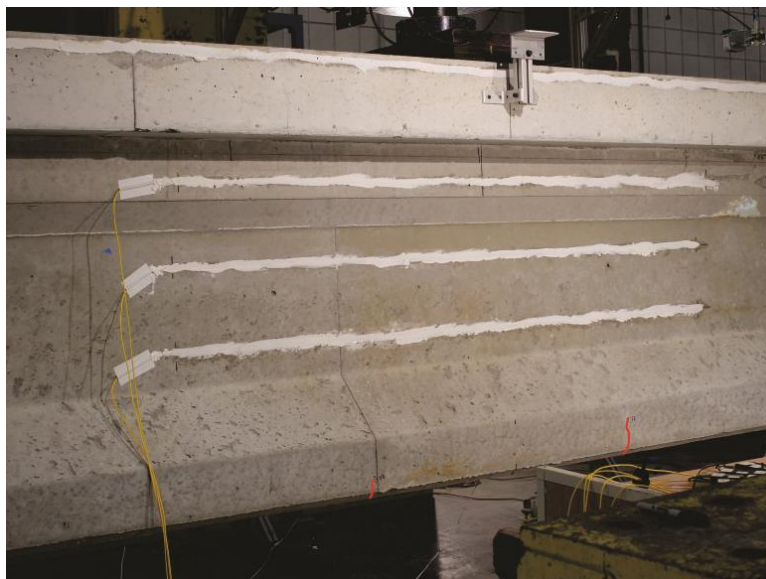
Figure 8.26 Specimen SS-2: First observed cracks (marked in red) at P = 77 kip
