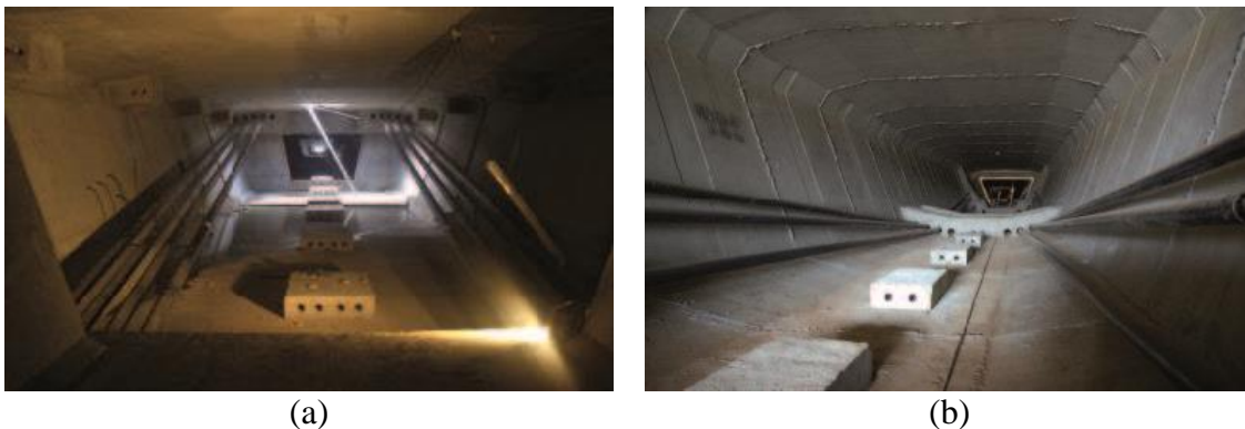
Figure 2.4 External tendons: (a) East Tsing Yi Viaduct, Hong Kong, (b) Gautrain Rapid Rail Link, South Africa (VSL International Ltd., 2009)
