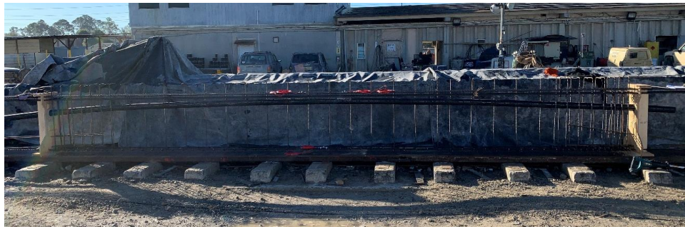
Figure 7.6 Rebar cage and HDPE duct installation for NB precast beams (before the ducts were tied for final configuration of tendon profile)
