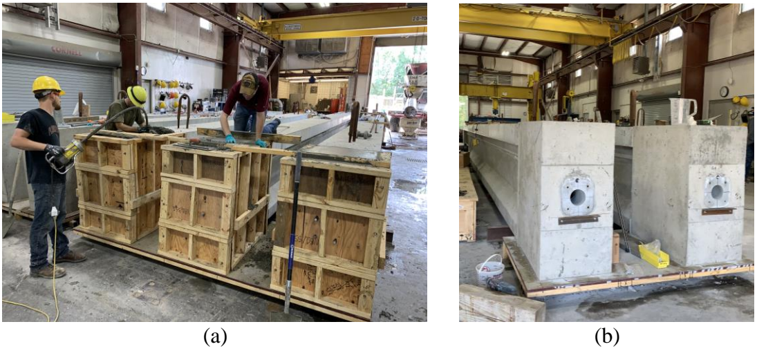
Figure 5.22 Fabrication of end blocks: (a) concrete placement; (b) end blocks (SS-3 and SS-4) after removal of formwork
