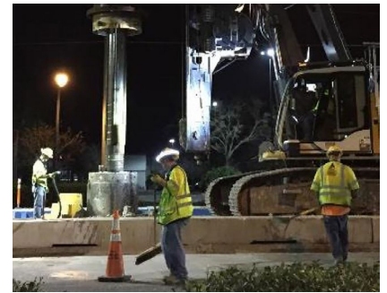
A construction crew operates a drill rig at night on the Selmon Parkway in Tampa.
