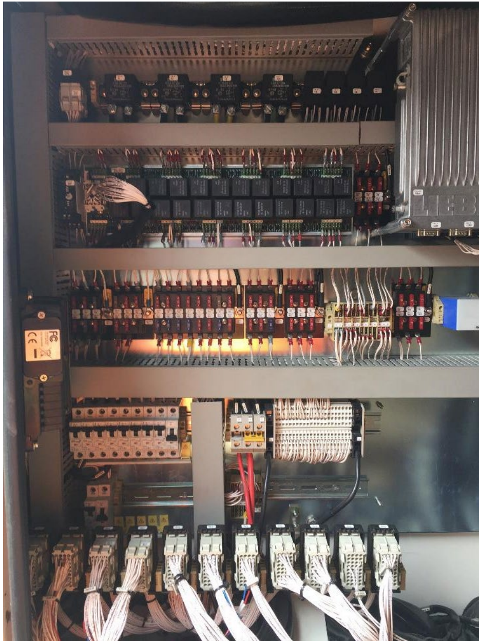
Figure 2-3. Liebehrr electrical unit.
