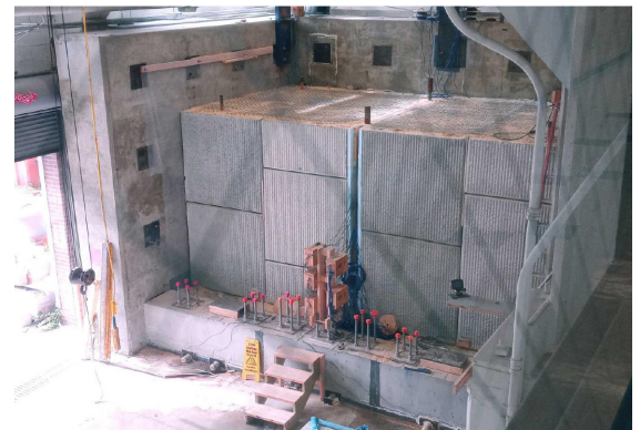
An overview of the completely constructed MSE wall area prior to load testing.
