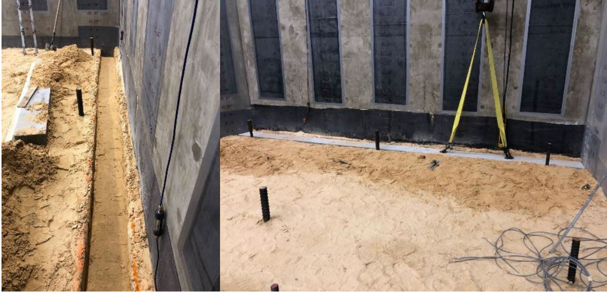
Figure 4-11. Cutting trenches in the base layer for leveling pads and placing the leveling pads.
