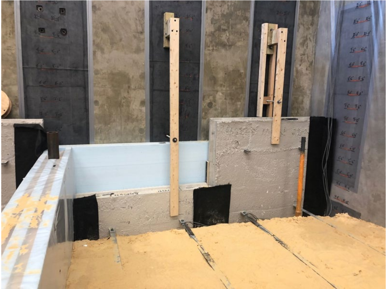
Figure 4-23. Frist row of reinforcement strips with filter cloth placed in the joints of wall panels.
