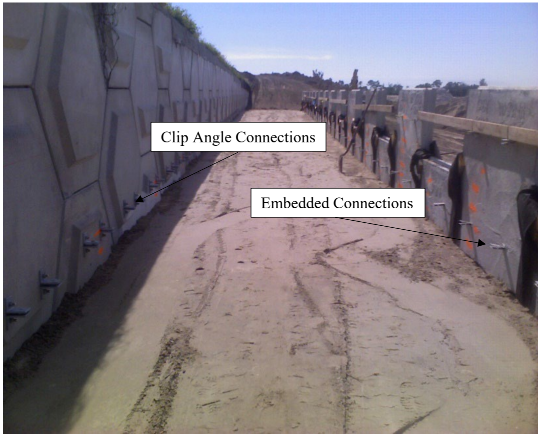
Figure 3-2. Back-to-back wall construction displaying embedded and clip angle connections that will both be mechanically fastened to the respective reinforcement.
