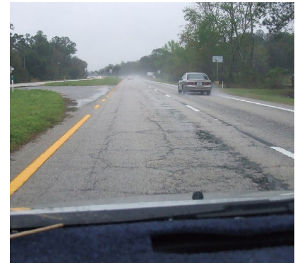
Load-induced fatigue damage appears as a network of cracks that become denser, leading to loss of asphalt.
