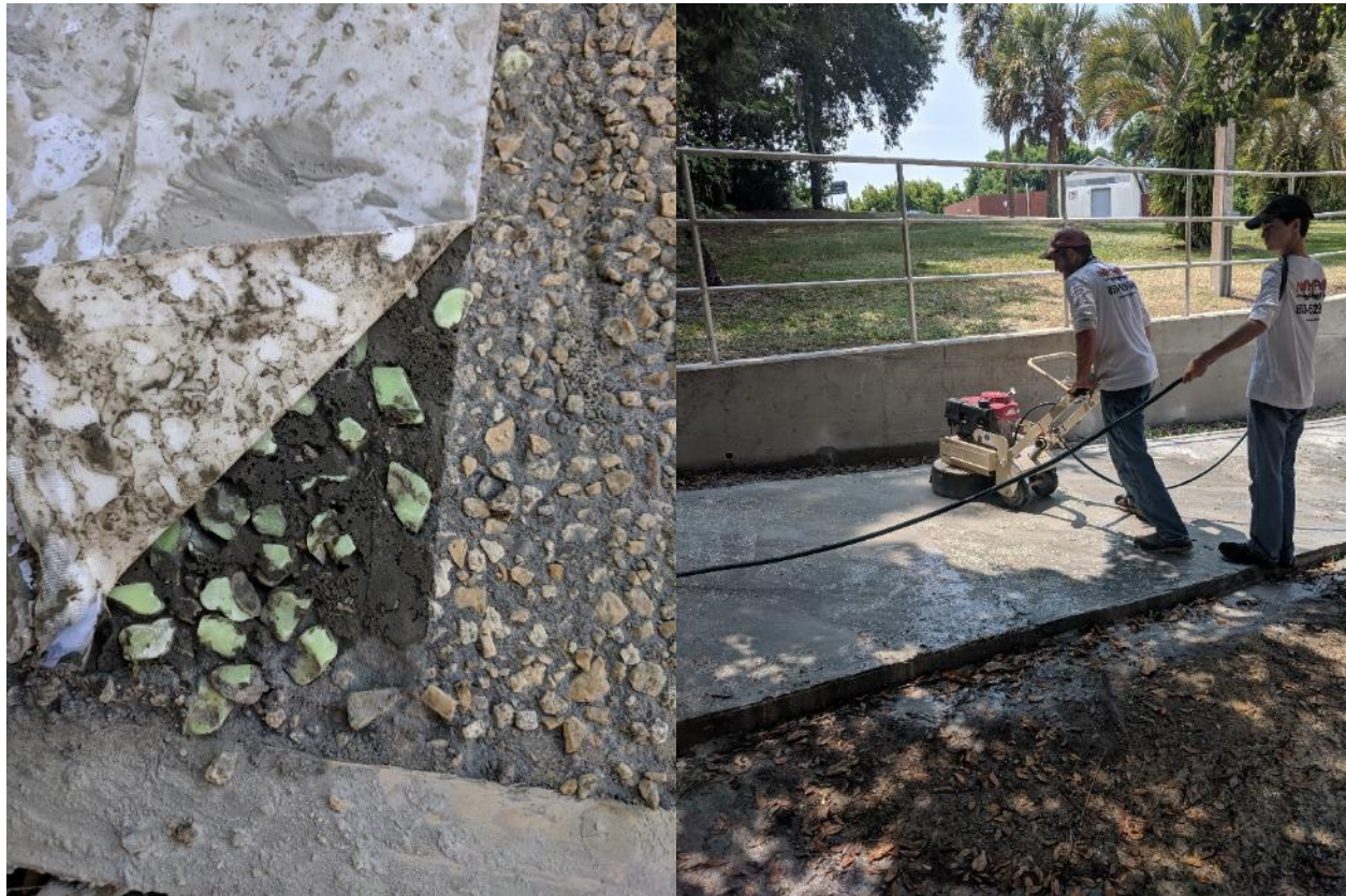
Figure 5-4. One week later, the tape backing was removed, and the stones were mostly well integrated but there were sections that did not adhere well to the concrete because it cured for too long (left). Contractor using polishing machine to smooth elevated and uneven sections (right).
