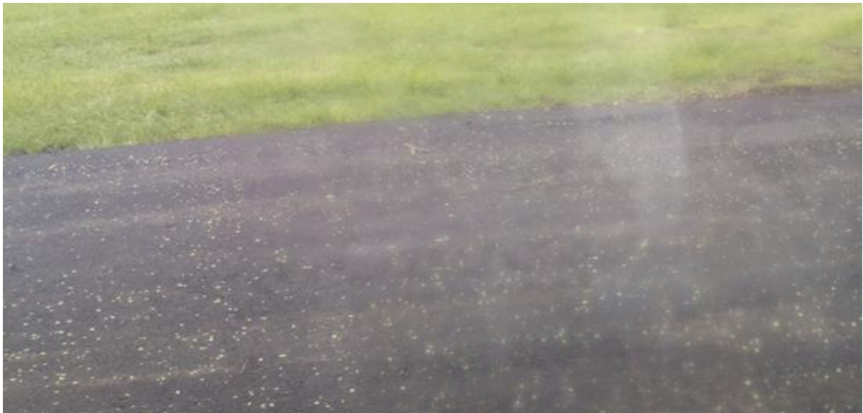
Figure 4-40. Image taken on June 15 th , 2019 from within the weatherproof enclosure installed at the asphalt pathway.
