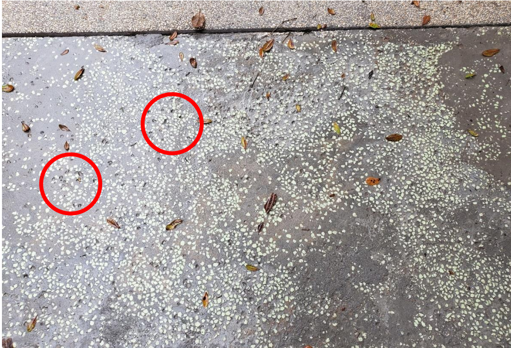
Figure 5-36. In this section of the installation, prefabricated sheets were used and then everything was sanded and ground down to make the surface smooth. In general, the glowing stones are all well integrated, but some were removed after the back covering was peeled away. Selected sections where stones are removed are indicated with the red circles.
