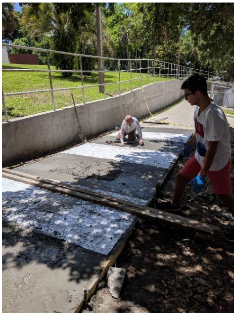
Figure 5-3. The pre-fabricated logos were placed under the concrete by the contractor. Solid sections of carpet tape were flipped, and the bottom, white side is shown. These sections were smoothed but not covered by concrete.
