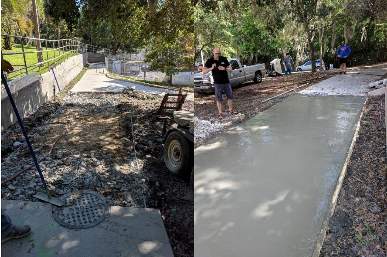
Figure 5-2. Sidewalk after removal of prior (left) and sidewalk after pouring concrete (right).
