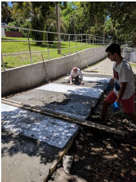
Figure 5-3. The pre-fabricated logos were placed under the concrete by the contractor. Solid sections of carpet tape were flipped, and the bottom, white side is shown. These sections were smoothed but not covered by concrete.
