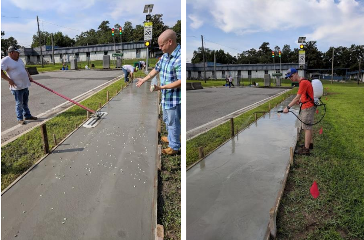
Figure 4-17. Sprinkling stones, followed by smoothing with a trowel (left) and spraying a retardant solution on the top, smoothed surface (right).
