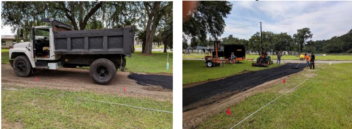
Figure 4-21. Truck used to transport and unload asphalt (left) and smoothing of asphalt by hand after unloading from the truck (right).
