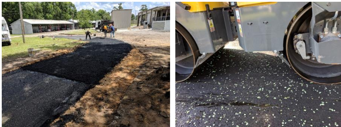
Figure 4-23. Contractors smoothing the last section of the installation (left) and a glimpse of the embedded stones underneath the smoother (right).
