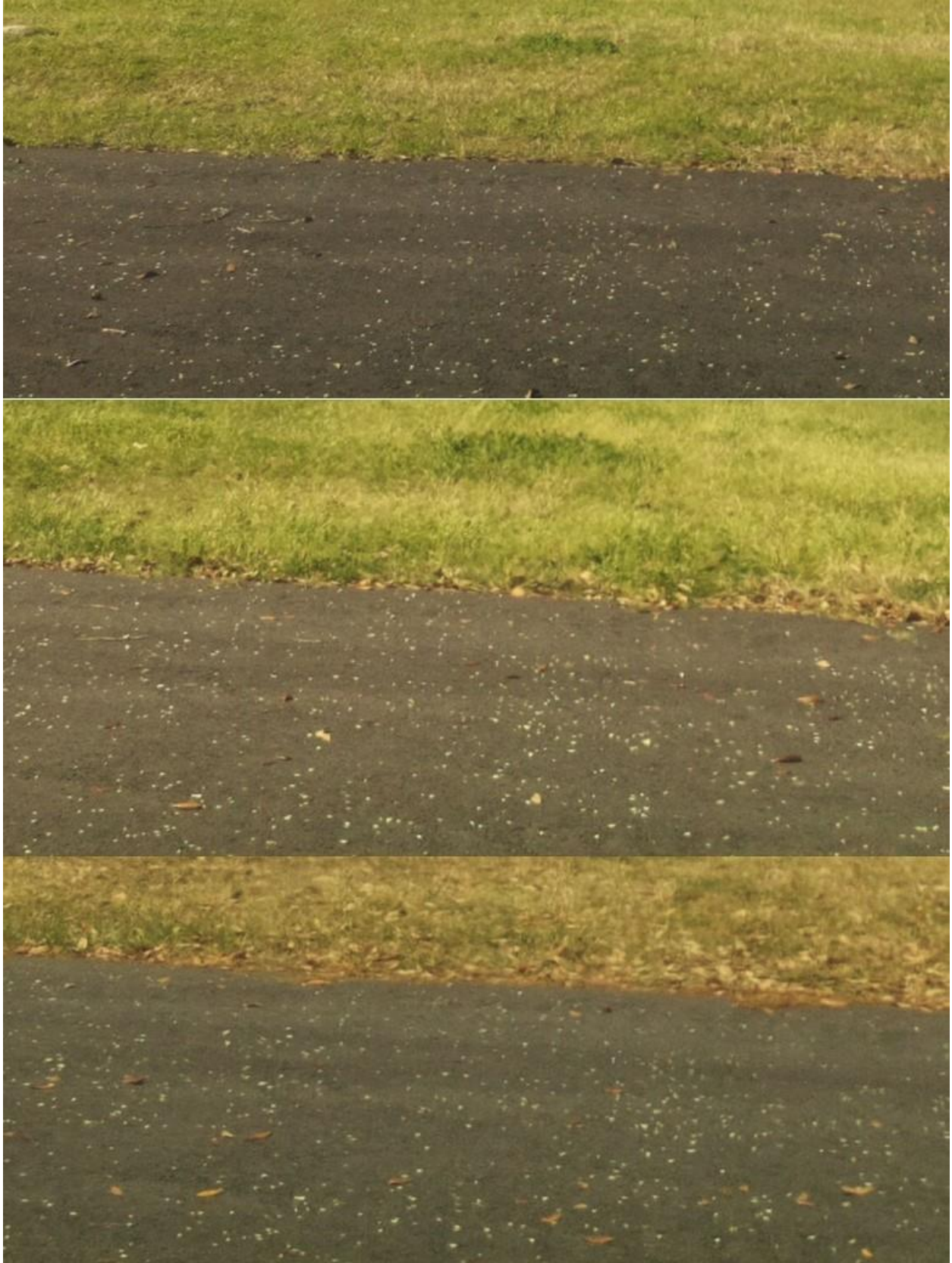
Figure 4-41. Images taken from within the weatherproof enclosure installed at the asphalt pathway on 12/22/2018, 2/21/2019, and 4/03/2019.
