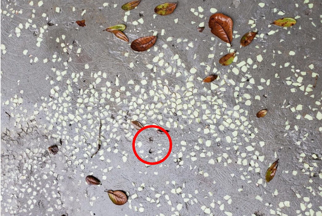
Figure 5-37. A zoomed in look at one of the areas where stones were not well integrated.
