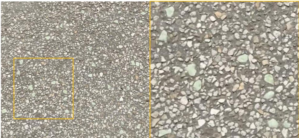
Figure 4-45. Top-down view and zoomed-in images of the concrete. Glowing stones can be recognized by their larger size, compared to the other exposed aggregate particles. Although only a single area is shown, this is representative of the entire installation. No attrition or raveling is observed, but the color of the stones has noticeably faded.
