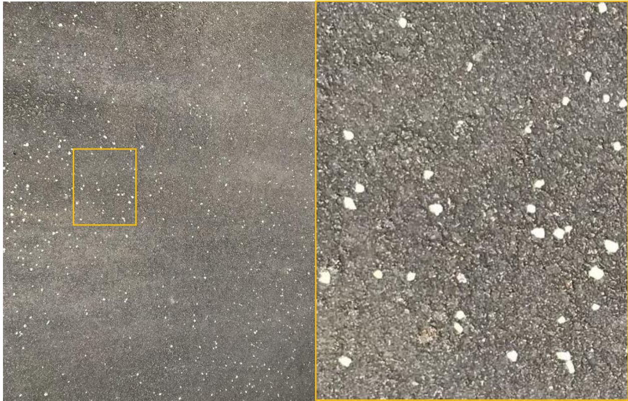
Figure 4-42. Top-down view of the asphalt installation (left). Zoomed-in image showing the integration of the stones in the asphalt (right).
