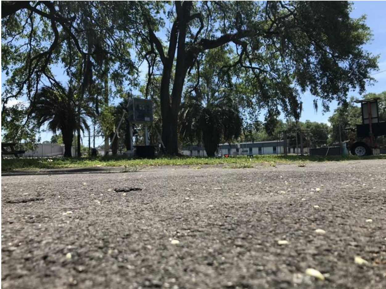
Figure 4-43. Horizontal image showing that the stone surface is level with surface of the asphalt.
