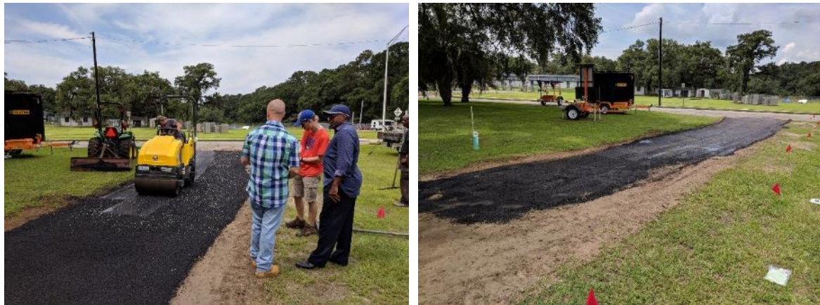
Figure 4-22. Roller smoothing asphalt with the stones integrated (left) and the asphalt after the first batch was unloaded and smoothed (right).
