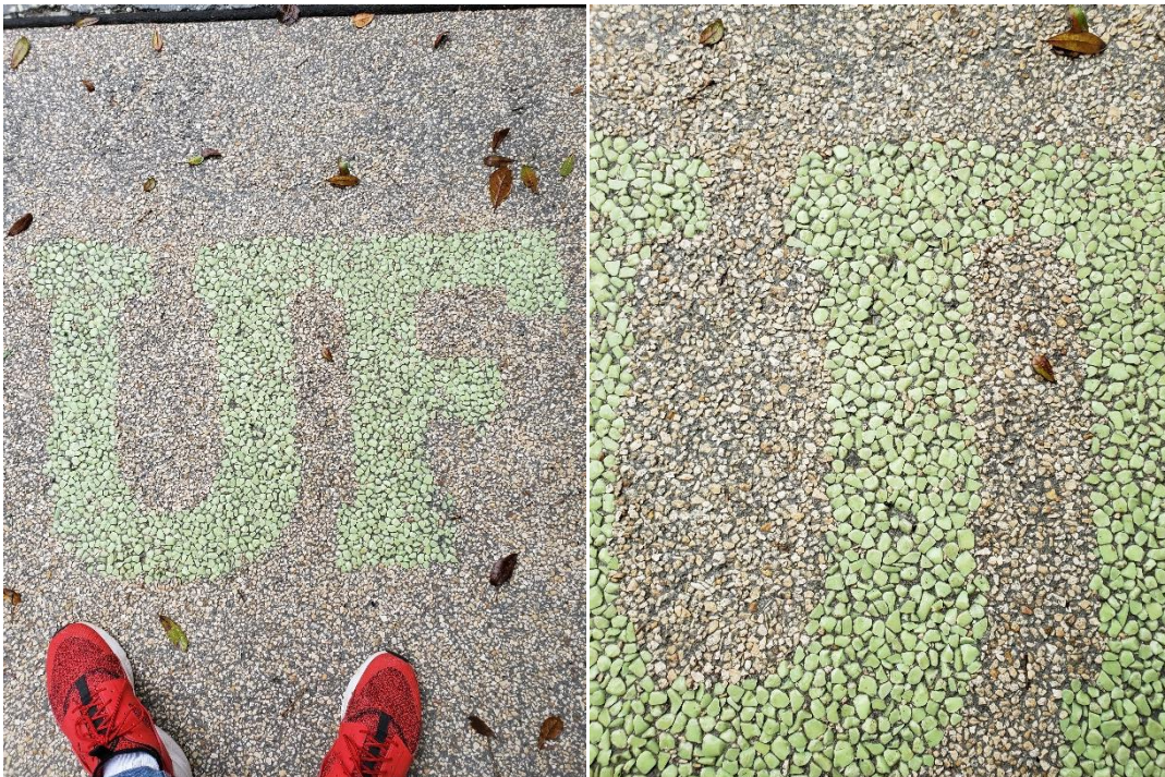
Figure 5-35. Stones that were placed while the concrete was still wet are showing no sign of attrition.
