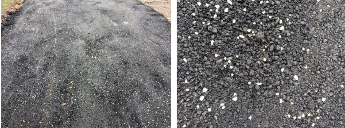
Figure 4-24. Zoomed-out images showing the “cold-rolled” areas that do not look homogeneous (left) and a zoomed-in image of one of these areas (right). In the “cold-rolled” sections the stones were not embedded well (right).
