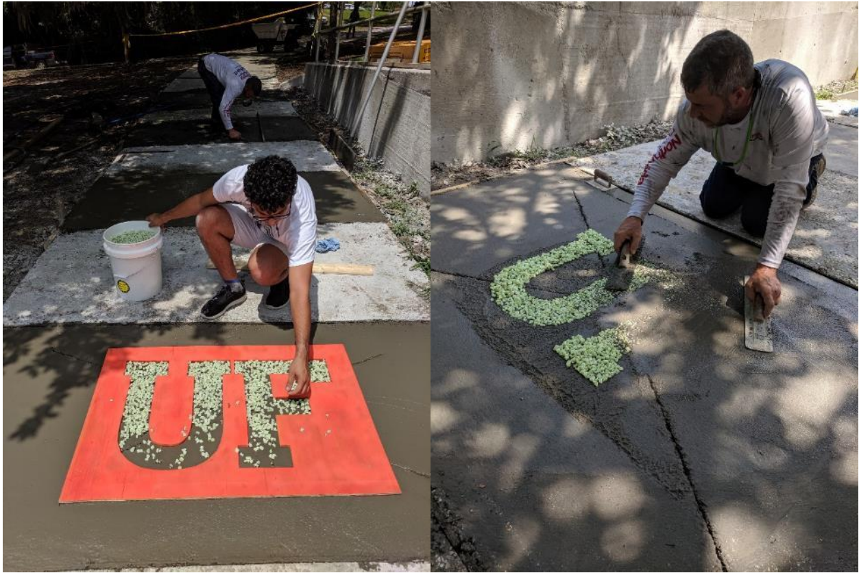
Figure 5-6. Stencil used to create the UF logo out of glowing stones (left). Contractor using a trowel to embed the stones in the concrete (right).
