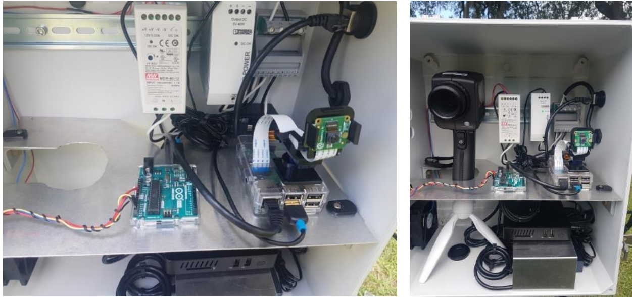
Figure 4-12. Final design on site without (left) and with luminance meter (right)
