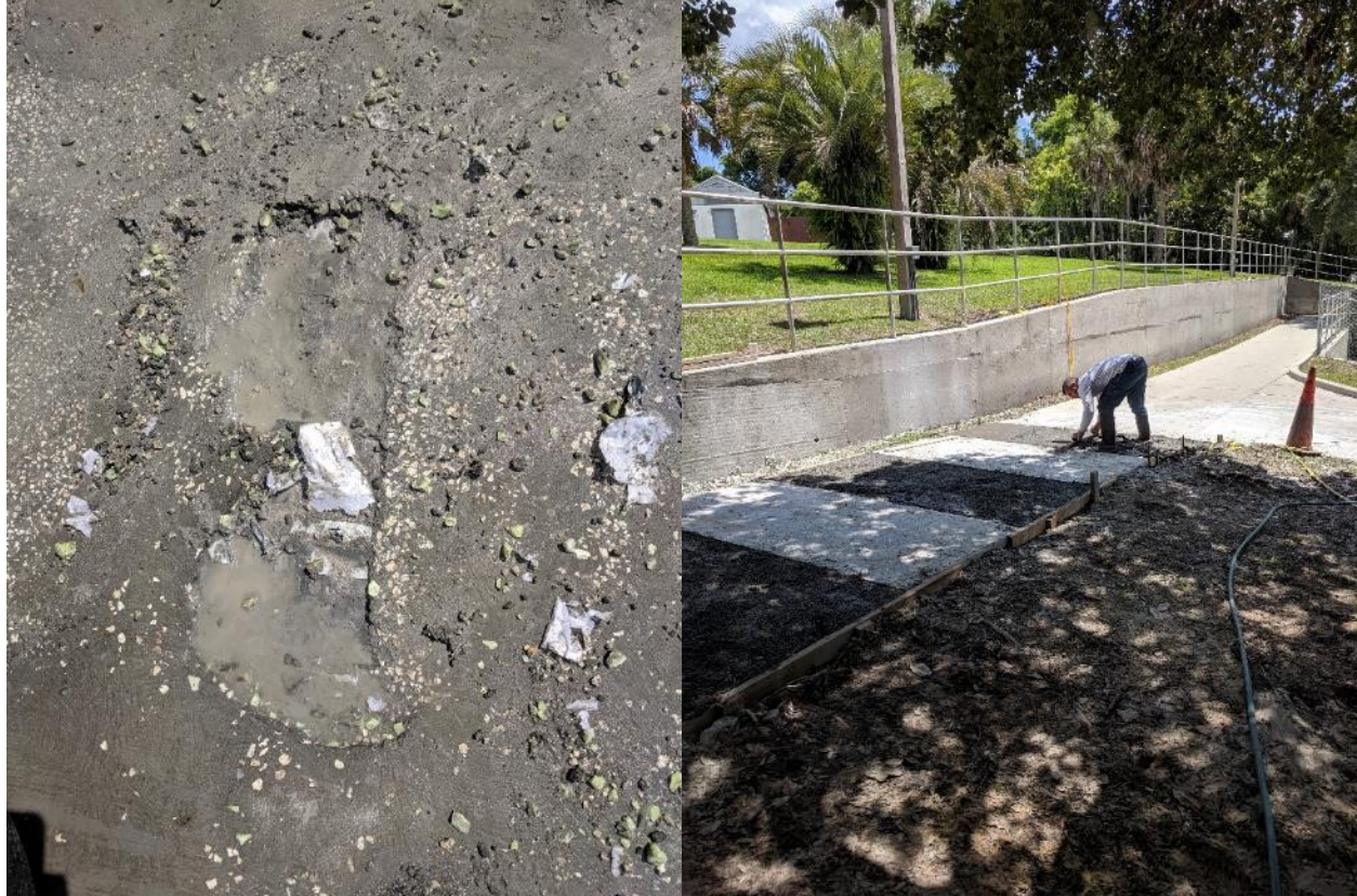
Figure 5-5. Representative image of the tape that was caught in the polishing machine (left) and freshly poured concrete in the sections with logos that were removed (right).
