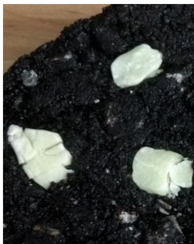
Figure 3-18. Cracked stones as a result of their large size and the compaction process.
