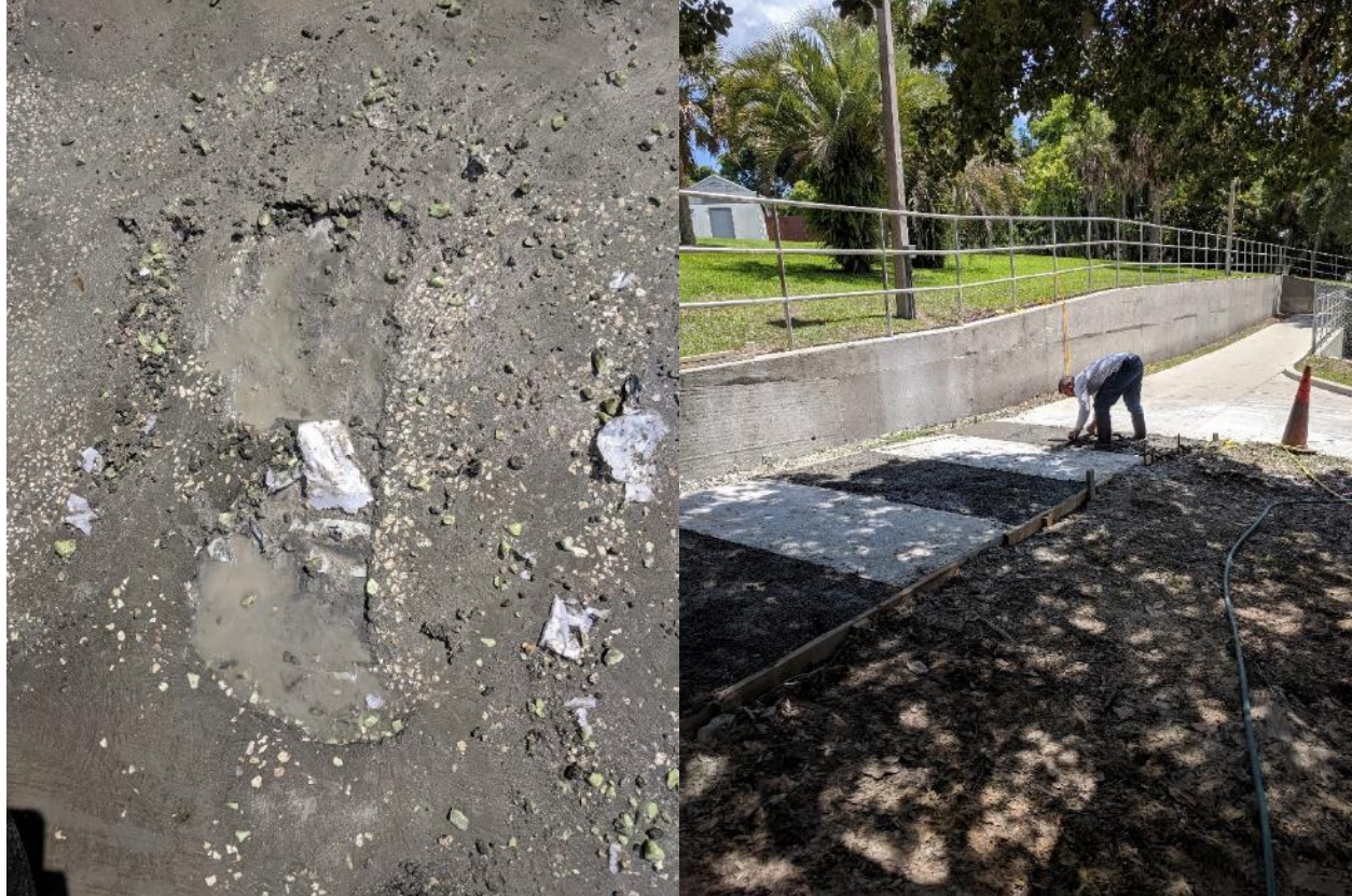
Figure 5-5. Representative image of the tape that was caught in the polishing machine (left) and freshly poured concrete in the sections with logos that were removed (right).
