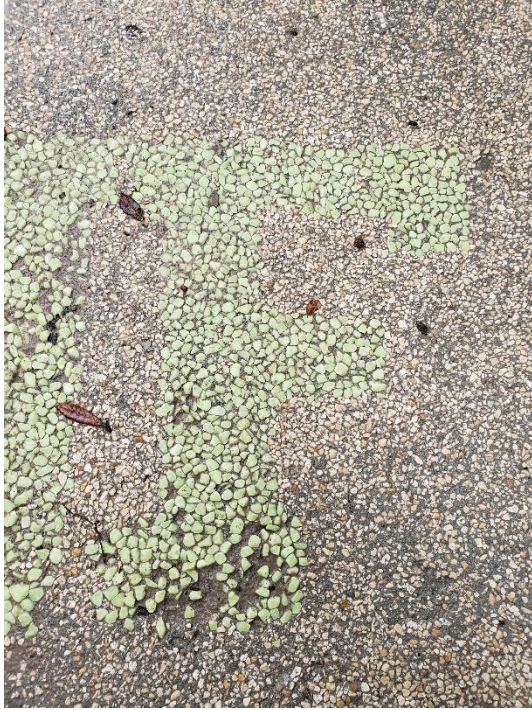
Figure 5-34. The last logo was placed after the concrete started to set, and some of the stones are coming loose.
