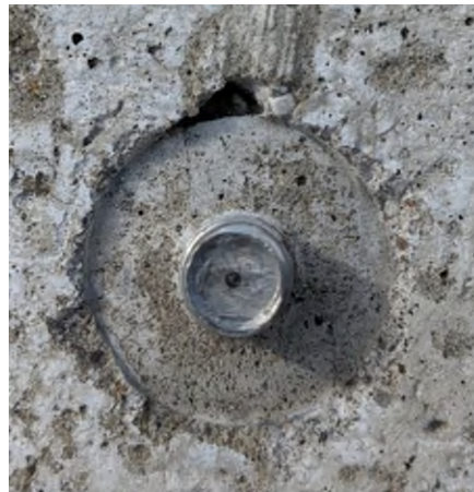
Figure 4-26: Gauge point created by drilling into threaded rod before embedding into concrete.
