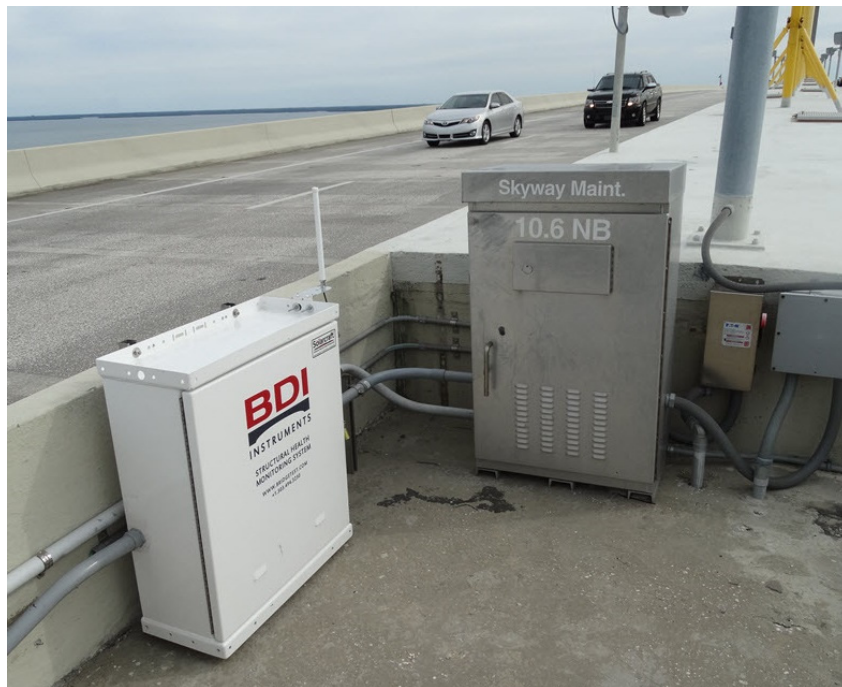
Figure 3. BDI data acquisition cabinet and DSMO maintenance cabinet
