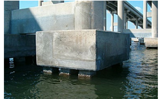
The concrete in this coastal bridge must withstand exposure to salt water for decades.
