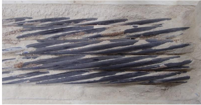
Figure 8-11. In situ corroded strands near port C dried TSG specimen
