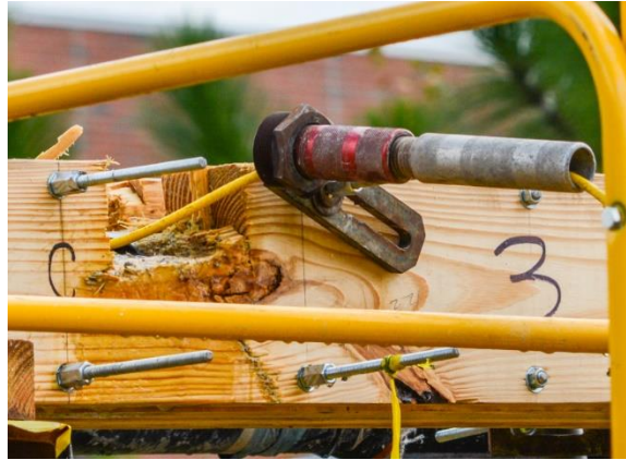
Figure A.4-4. Insertion of nozzle into the hole opening prior to hydrodemolition in trial 2
