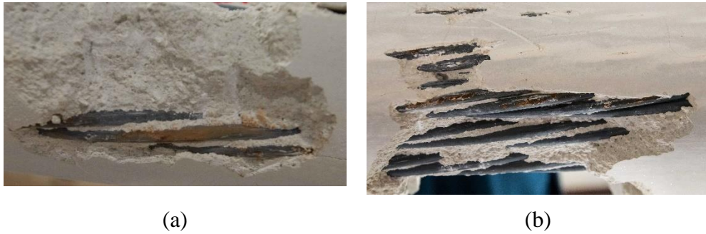
Figure 8-18. In situ corroded strands at: (a) port E; (b) port F dried ISG specimen
