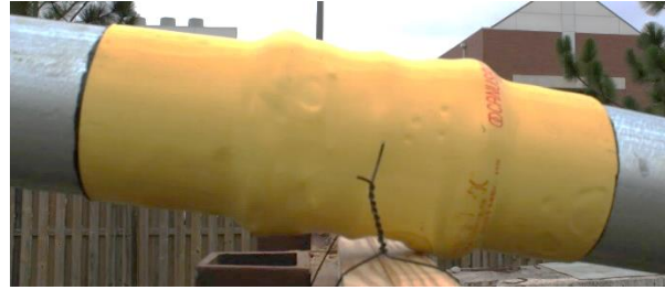
Figure A.2-4. Shrink wrap and coupler connecting two EMT sections
