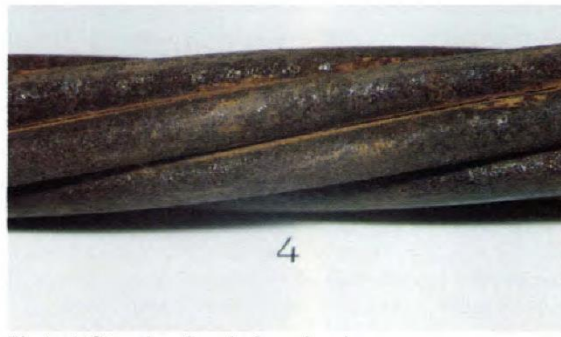
Photo 4. Strand surface before cleaning.
