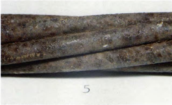
Photo 5. Strand surface before cleaning.
