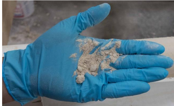
Figure 8-6. Soft grout crumbled with hand
