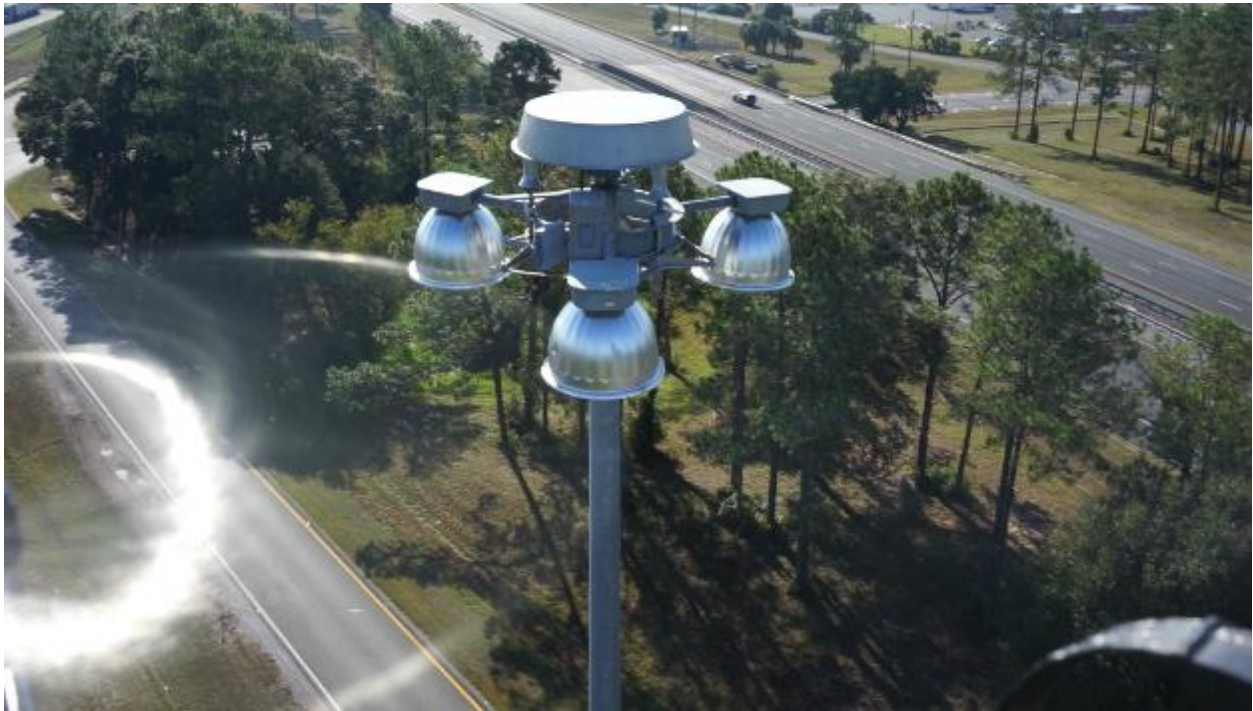
Figure A2-12. 32P050 - View of Lights from Northwest
