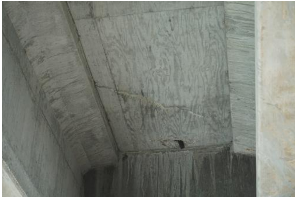
Figure A2-73. 790152 – View of spall in deck underside
