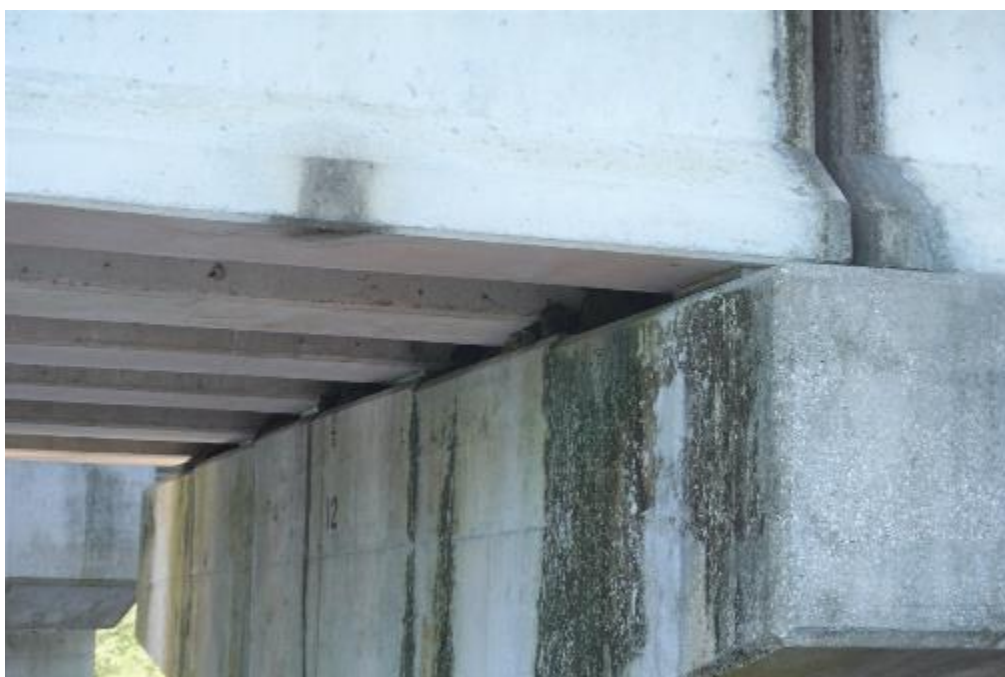
Figure A2-77. 300031 – Typical view of pier cap taken from outside of bridge
