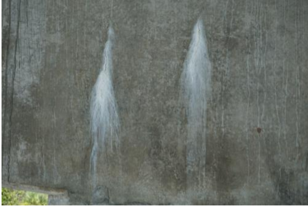
Figure A2-61. 790148 – Close up view of cracking with efflorescence in pier cap
