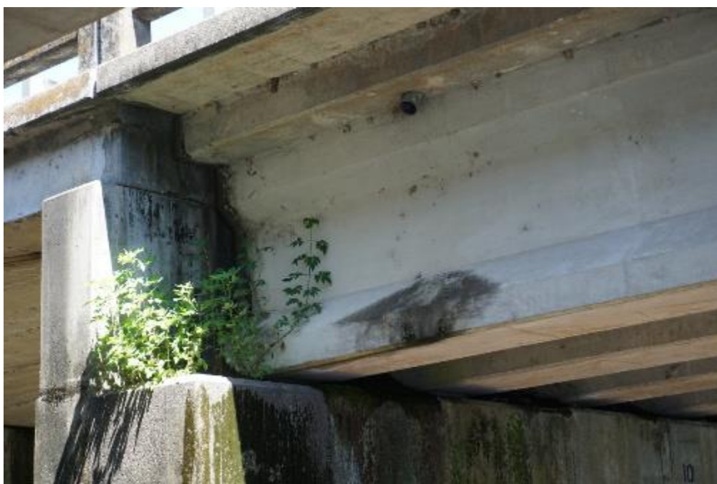
Figure A2-79. 300031 – Typical view of debris growth on pier cap
