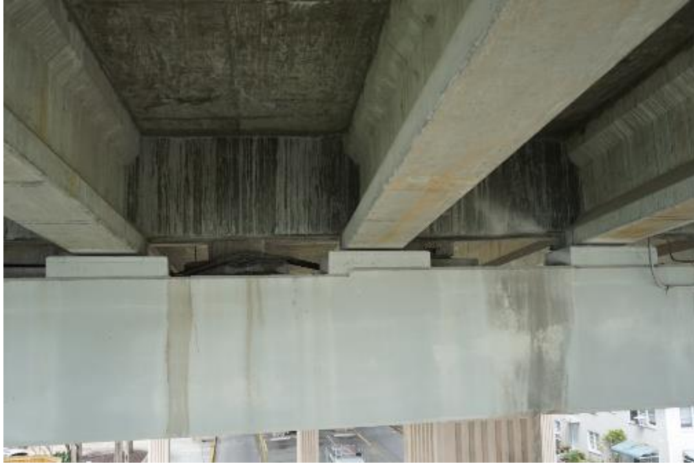
Figure A2-70. 790152 – View of debris on pier cap
