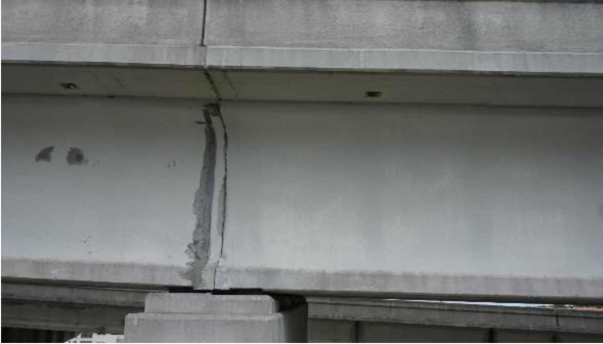
Figure A2-54. 720690 – Exterior view of prestressed concrete girders over a pier cap
