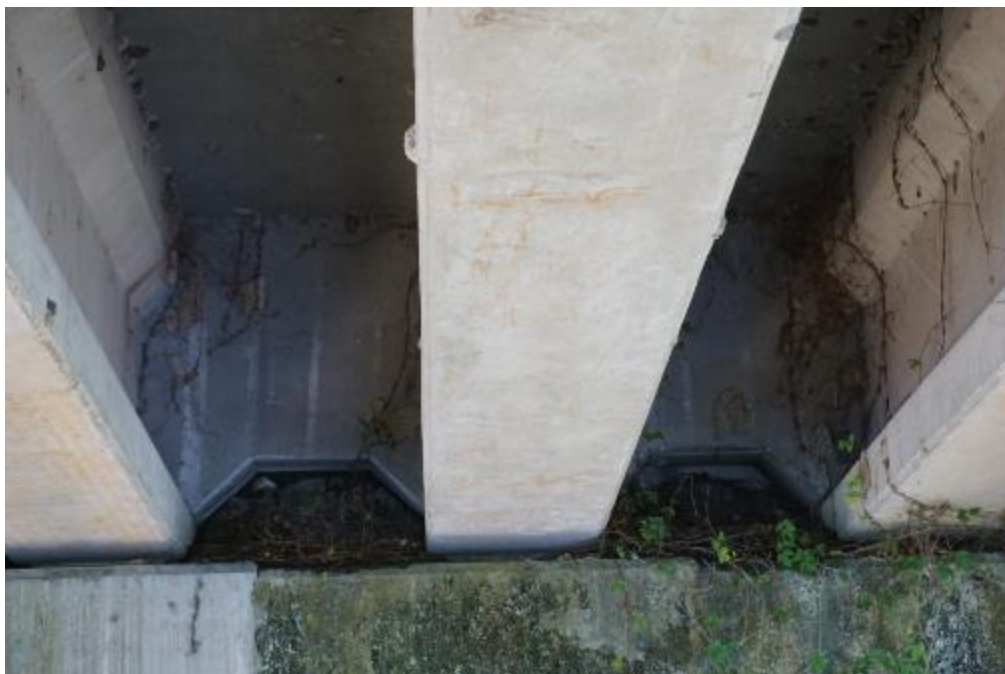
Figure A2-78. 300061 – Typical view of vegetation growth and debris on top of pier cap
