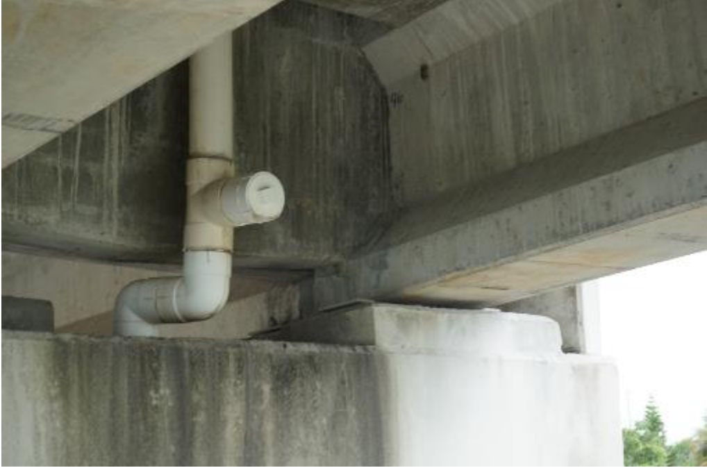
Figure A2-72. 790152 – Typical view of pipe above pier cap
