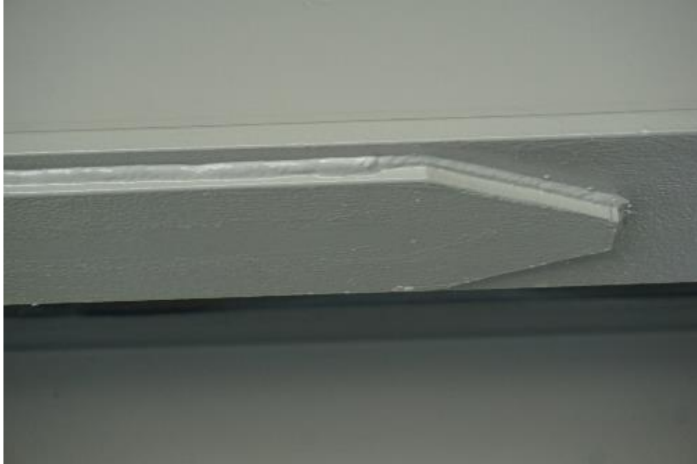
Figure A2-97. 290032 – Typical view of terminal of cover plate
