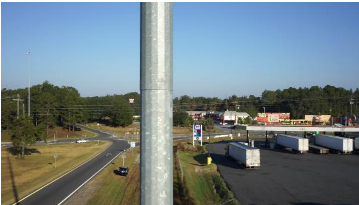
Figure 3-4. View of southeast face of first slip joint of 32P049
