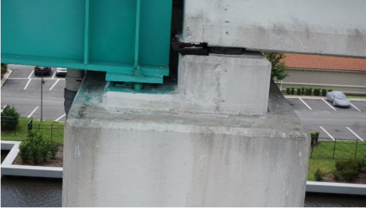
Figure A2-56. 720690 – Exterior view of steel and prestressed concrete girders over a pier cap
