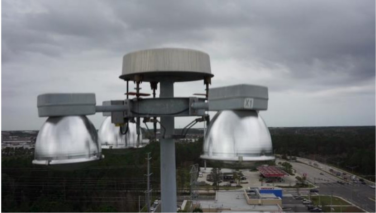
Figure A2-28. 72P740 - View of Lights from East
