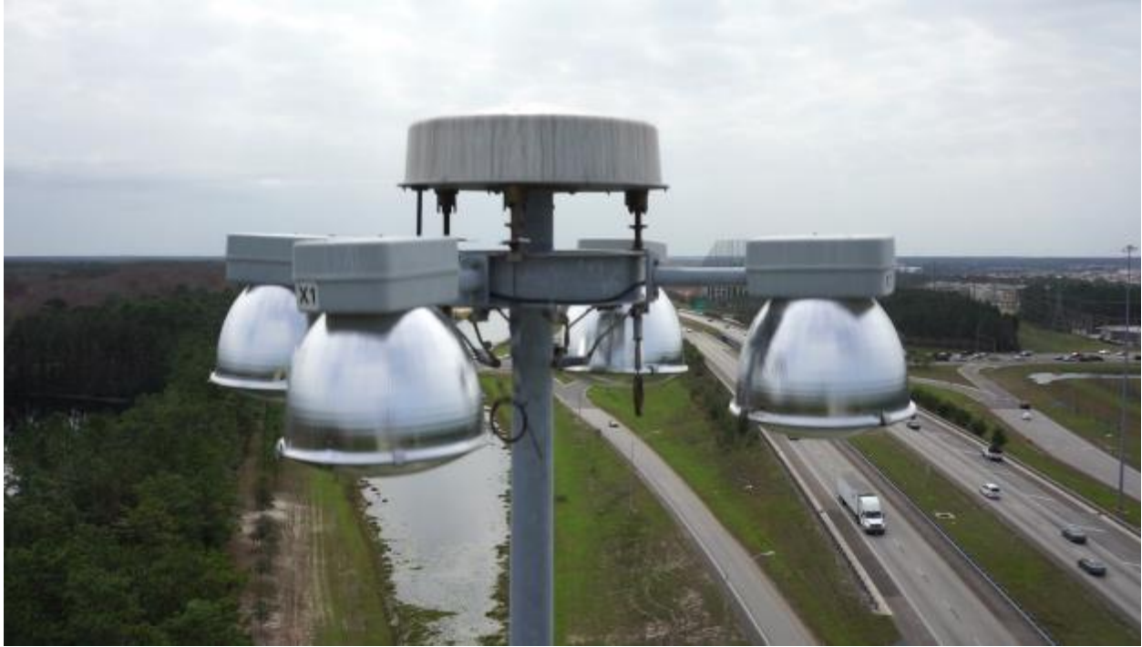
Figure A2-48. 72P743 - View of Lights from North
