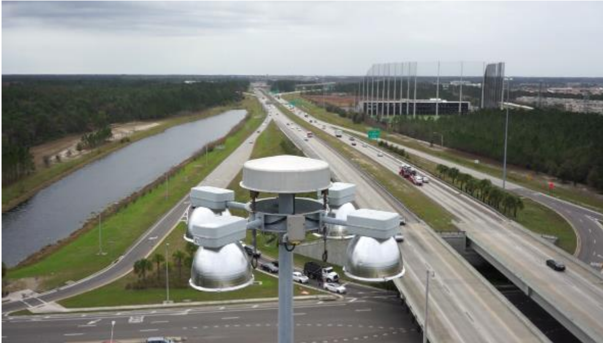
Figure 3-8. View of luminaire of 72P741 from north
