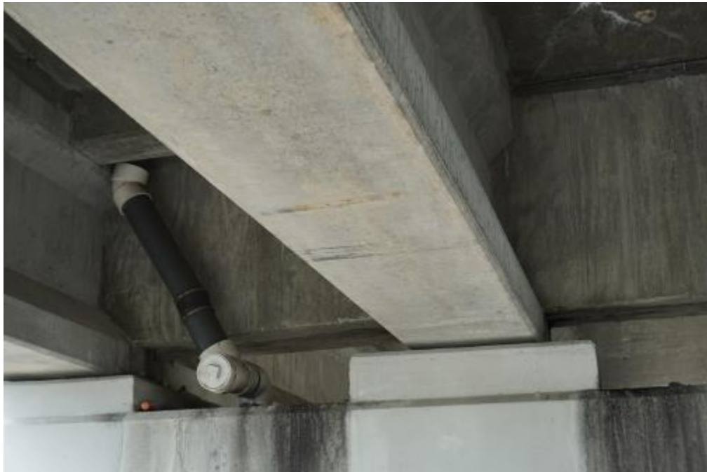
Figure A2-71. 790152 – Typical view of pipe above pier cap
