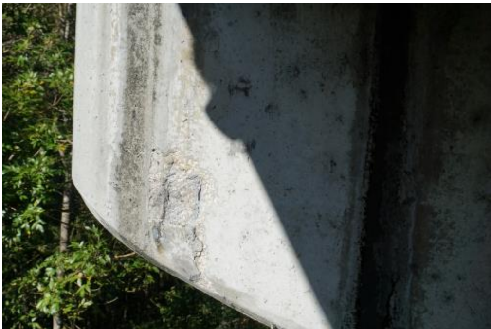
Figure A2-89. 360055 – View of spall in pier cap
