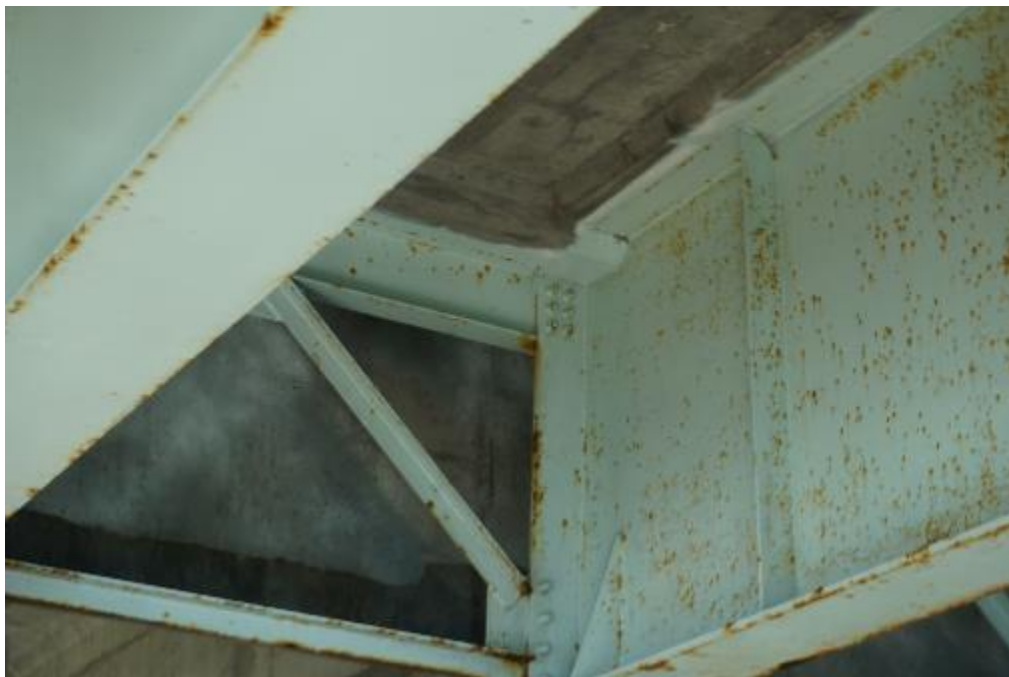
Figure A2-64. 790148 – Typical view of diaphragm connection to steel girder at beam end
