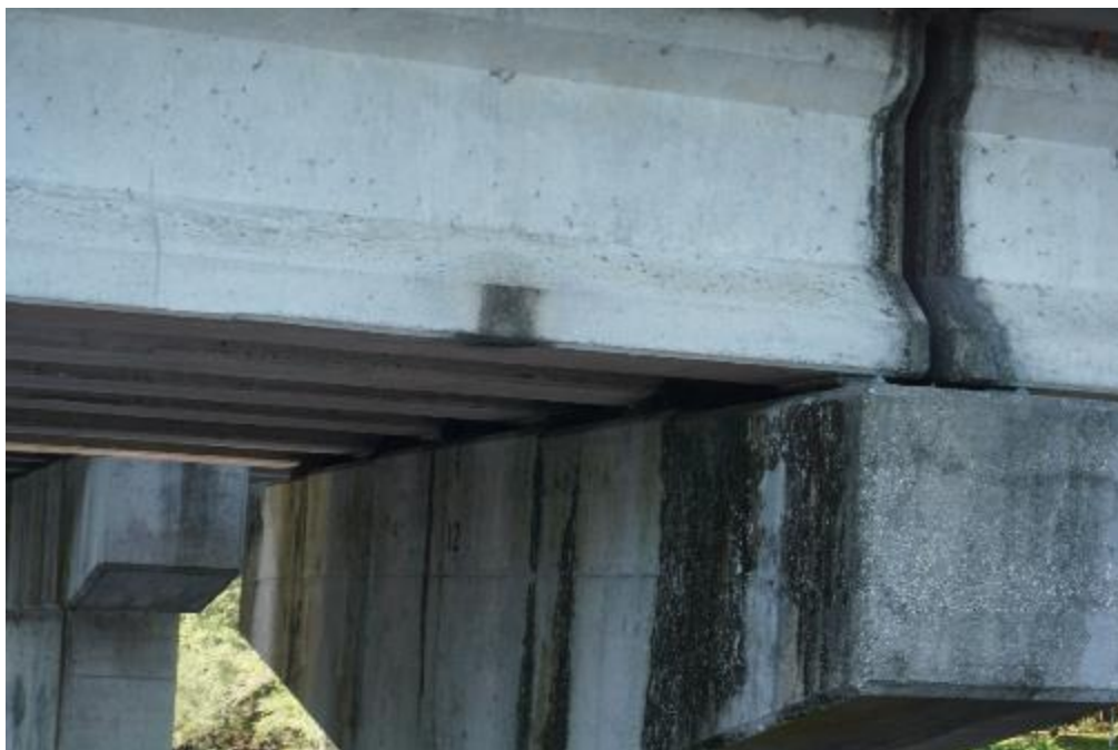
Figure A2-76. 300031 – Typical view of pier cap taken from outside of bridge
