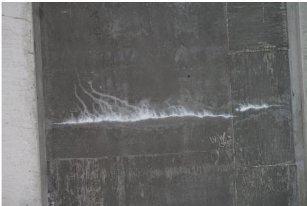
Figure A2-62. 790148 – Typical view of cracking with efflorescence in deck underside
