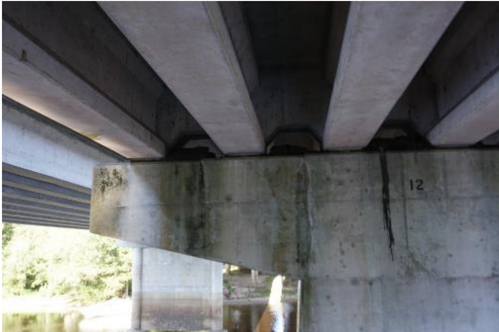
Figure A2-74. 300031 – Typical view of debris on top of pier cap
