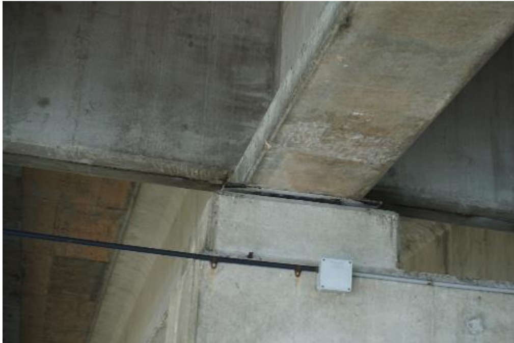
Figure A2-57. 790148 – Typical view of conduit with broken straps
