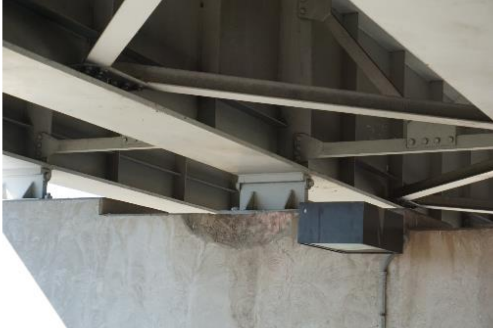
Figure A2-101. 720114 – Typical view of spall in pier cap underneath steel beam
