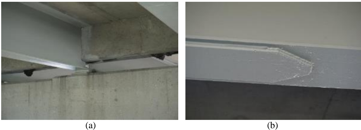
Figure 4-20. Sample images from inspection of 290032: (a) bearings and beam ends in Span 7 over Pier Cap 7, and (b) cover plate end in Span 5.
