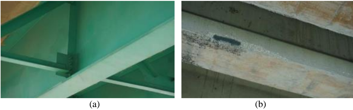
Figure 4-4. Sample images from inspection at 720044 and 720690: (a) connection of lateral bracing between beams in Span 9, 720690, and (b) spall on Beam 6-6, 720044
