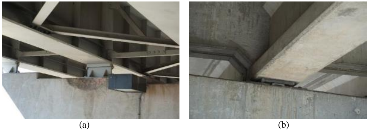
Figure 4-22. Sample images from 720114: (a) spall in Pier Cap 32 under Beam 32-7, and (b) bearing under a typical prestressed concrete girder.
