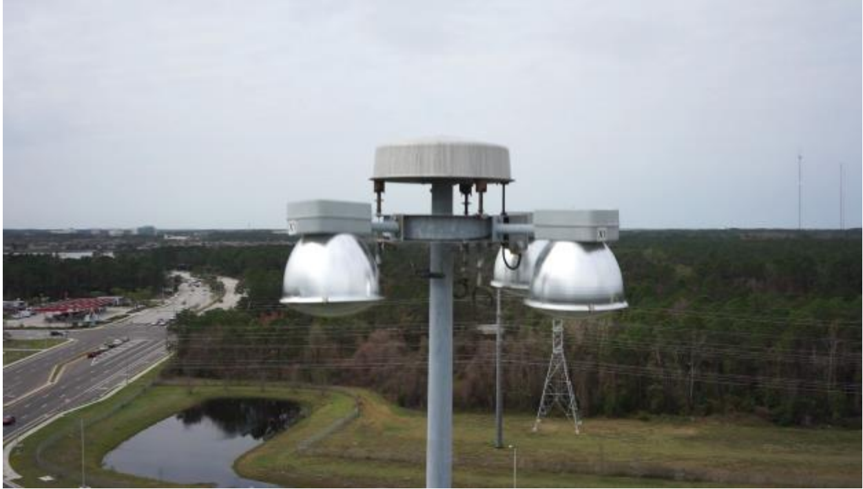
Figure A2-38. 72P741 - View of Lights from East
