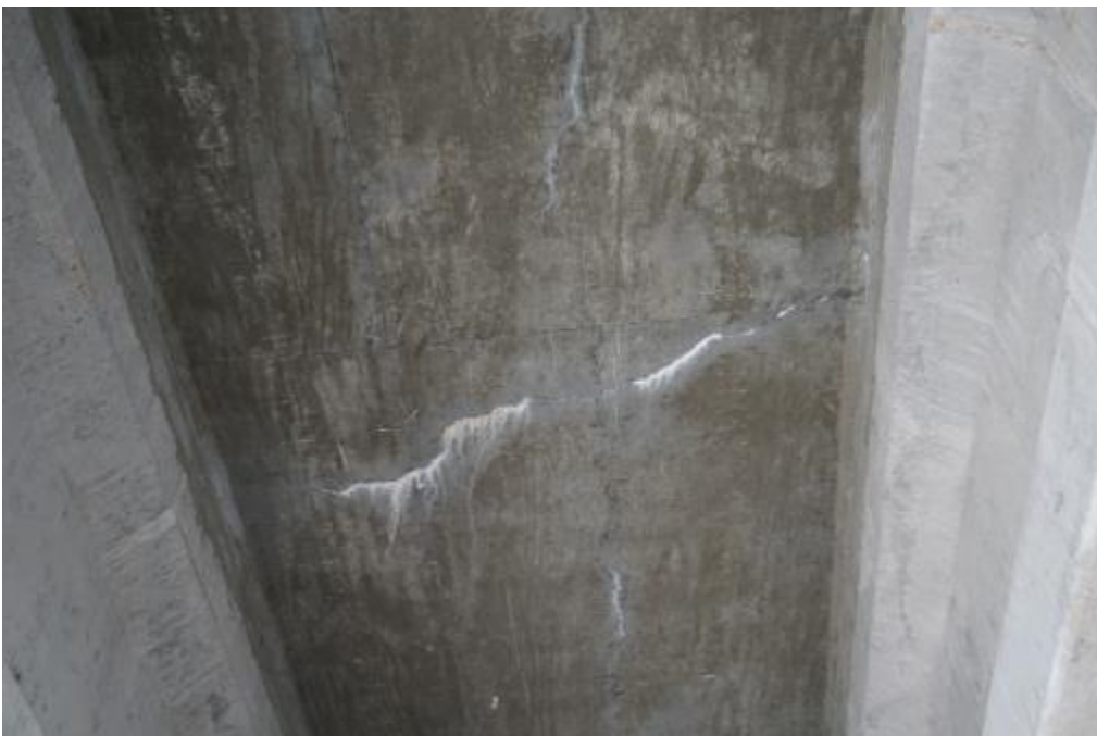
Figure A2-69. 790152 – Typical view of cracking with efflorescence in deck underside
