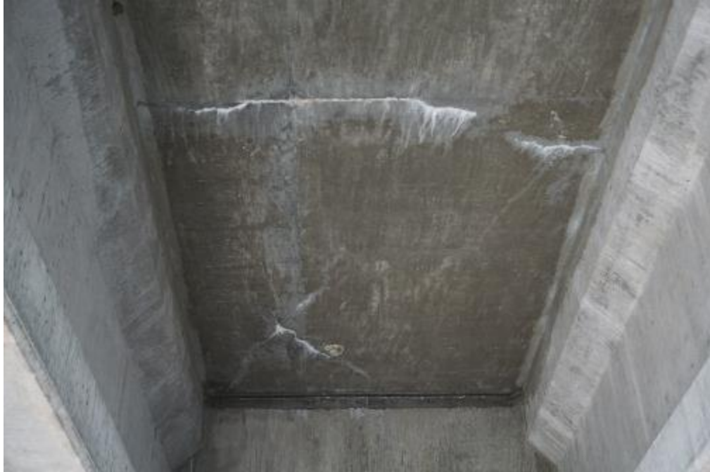
Figure A2-68. 790152 – Typical view of cracking with efflorescence in deck underside
