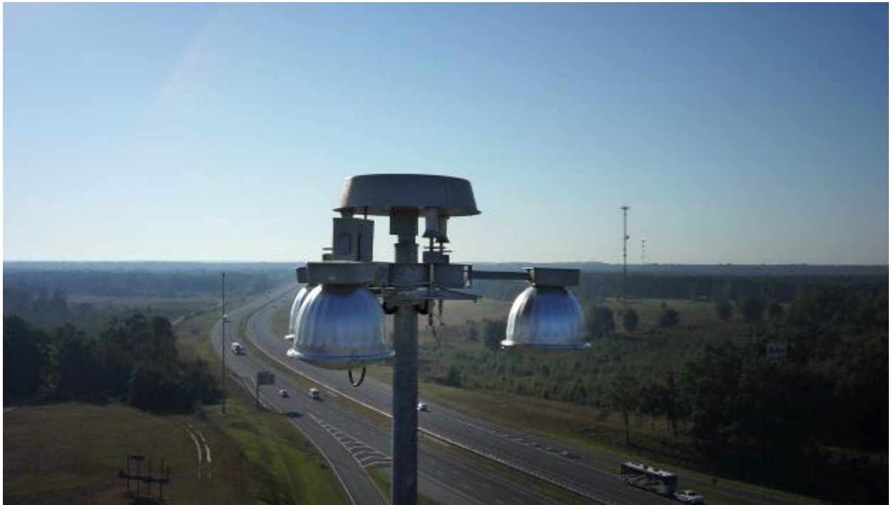
Figure A2-6. 32P049 - View of Lights from Northwest
