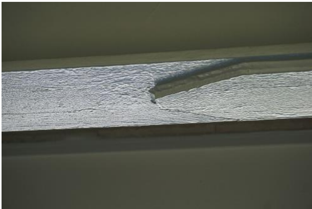
Figure A2-98. 290032 – Typical view of terminal of cover plate
