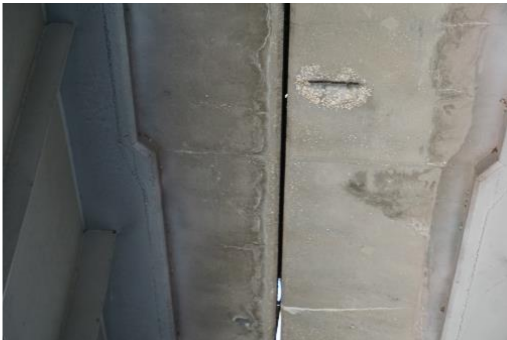
Figure A2-100. 720114 – Typical view of spall in deck underside
