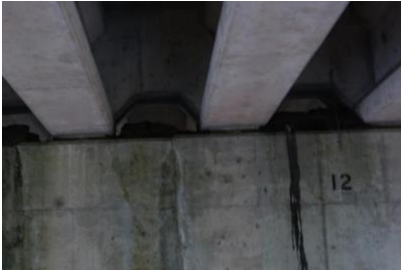
Figure 4-13. View of debris build-up on Bent Cap 12 of 300031
