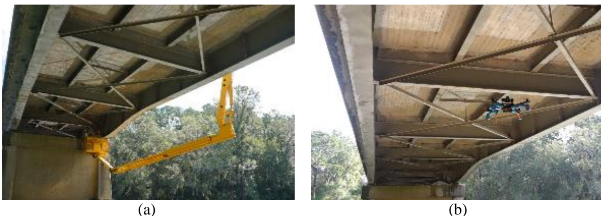
Figure 4-15. View underneath Span 4 of 320061: (a) UBIV routine inspection of Span 4, and (b) sUAV demonstration routine inspection of Span 4 conducted shortly after.
