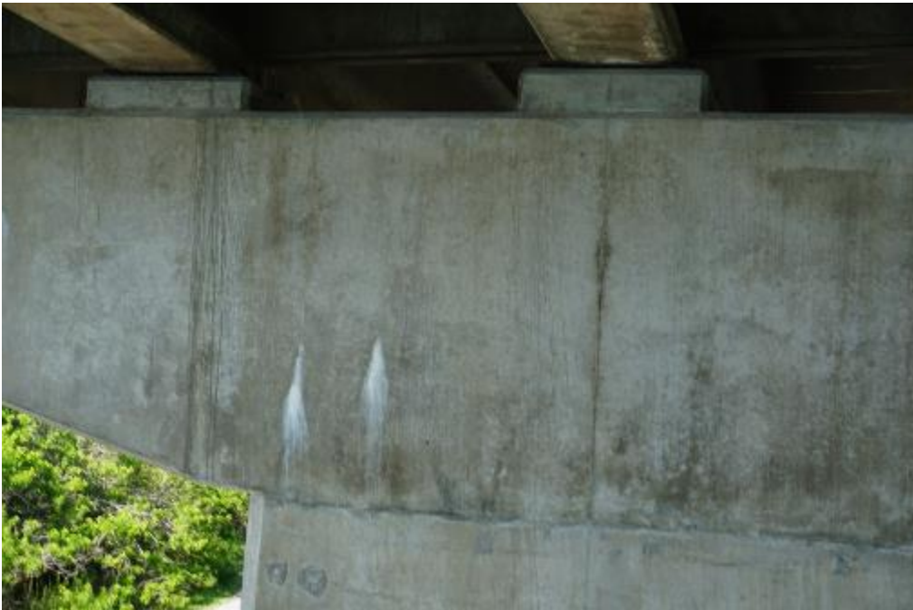
Figure A2-60. 790148 –View of cracking with efflorescence in pier cap
