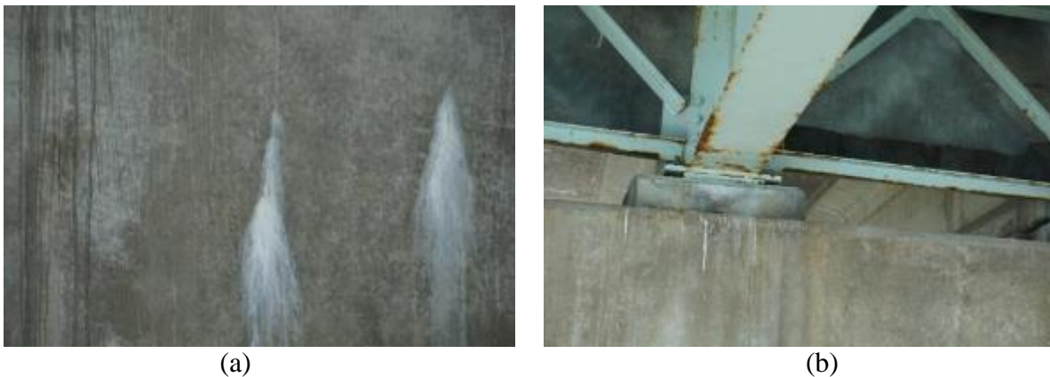
Figure 4-6. Sample images from inspection at 790148: (a) cracking with efflorescence in Pier Cap 4B, 790148, and (b) interior bearings in Span 7 over Pier 7
