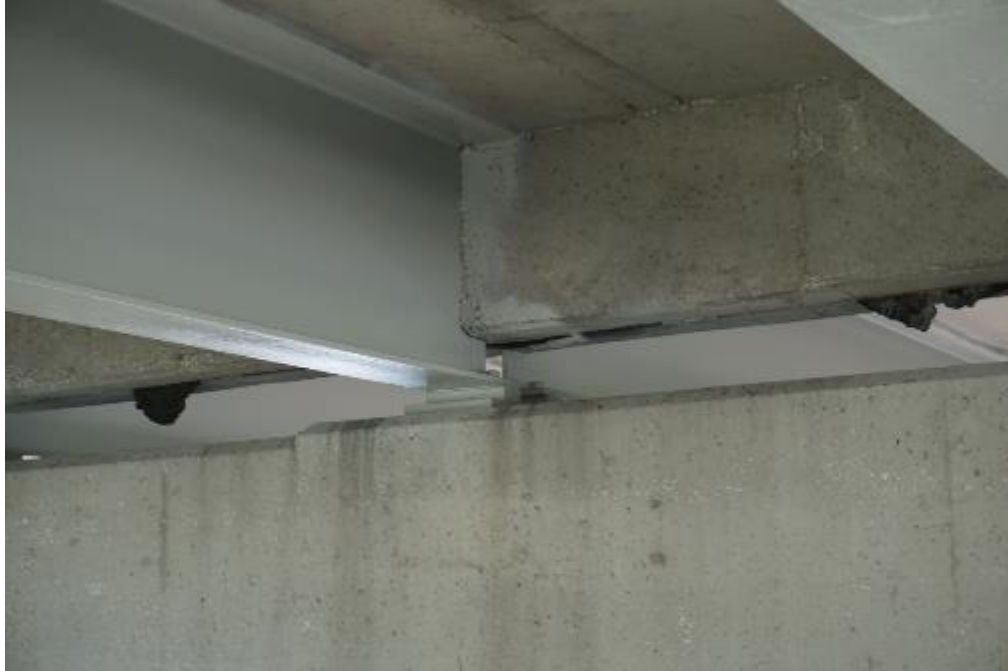
Figure A2-95. 290032 – Typical view of bearing under steel beam and steel beam ends
