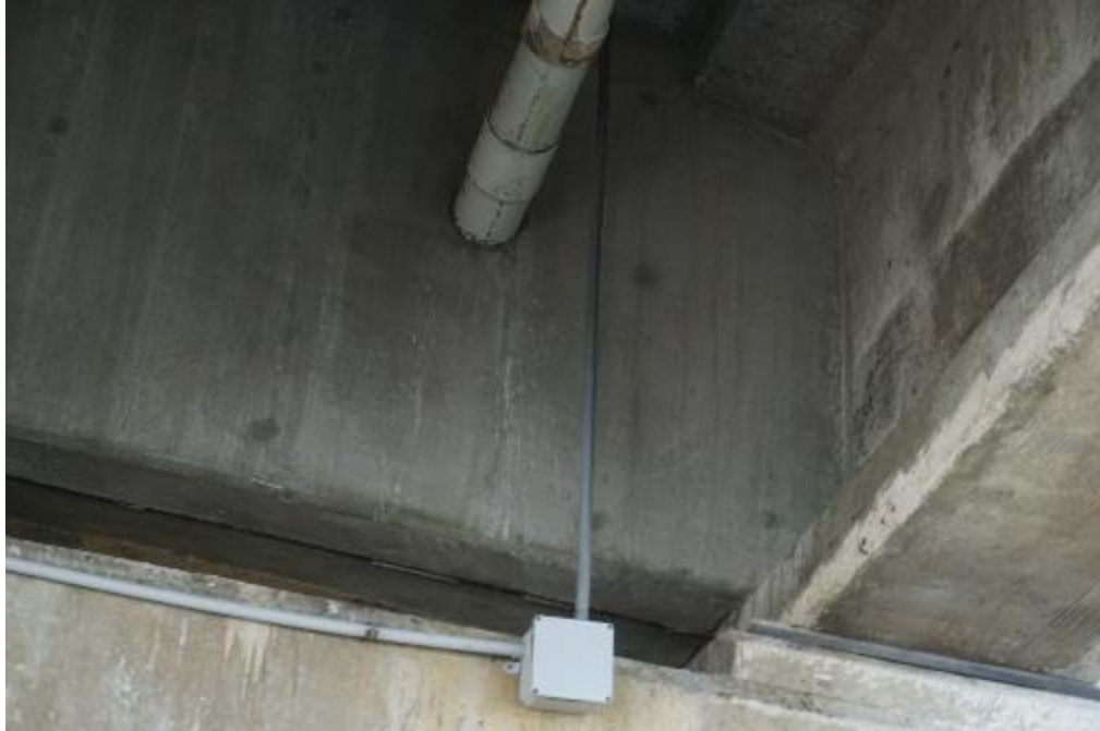
Figure A2-59. 790148 – Typical view of conduit
