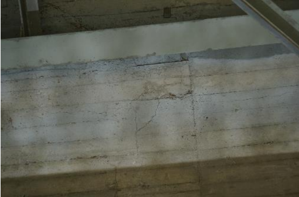
Figure A2-82. 320061 – Typical view of cracking in deck underside
