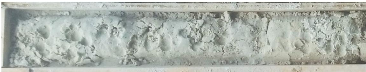
Figure 2-5. Weak, poorly cemented silt, sand, and limestone mixture in a core run
