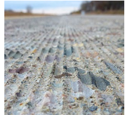
Grinding grooves into concrete pavement prepares it for a new top layer, but it generates tons of residual powder that must be properly disposed of.
