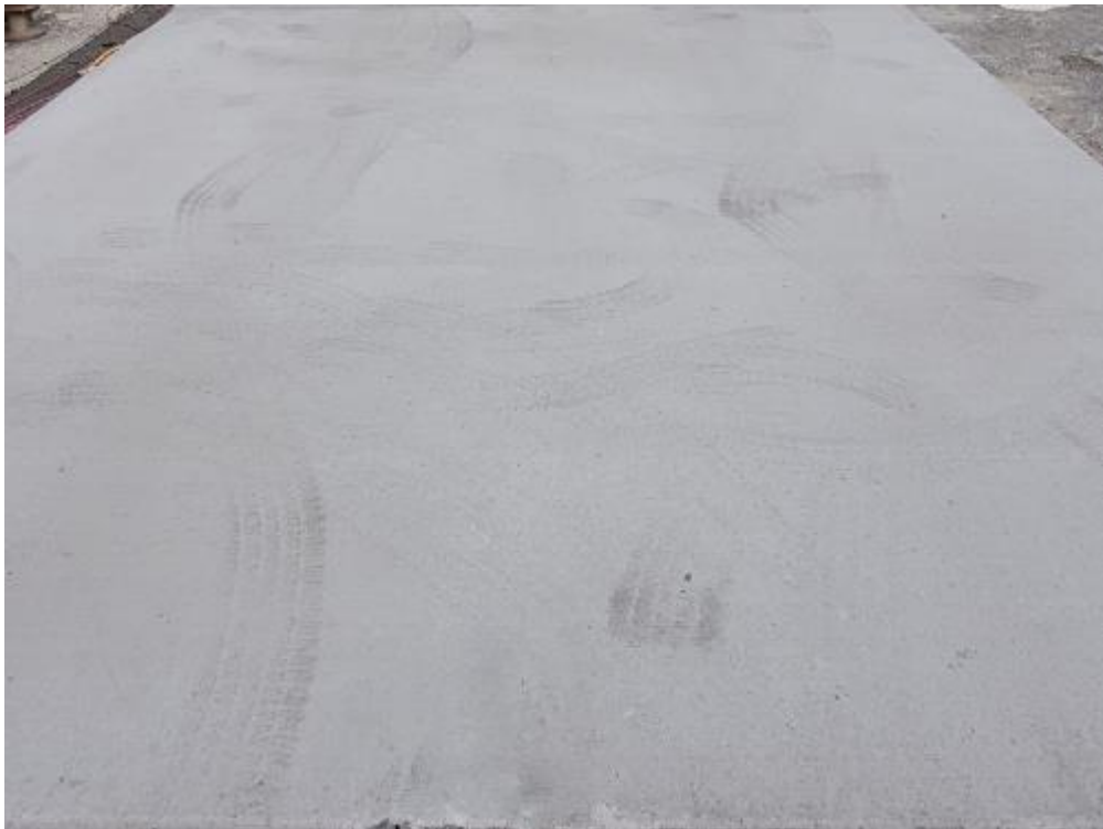
Fig 5.14 Picture of the surface of Slab3 ICC-2.
