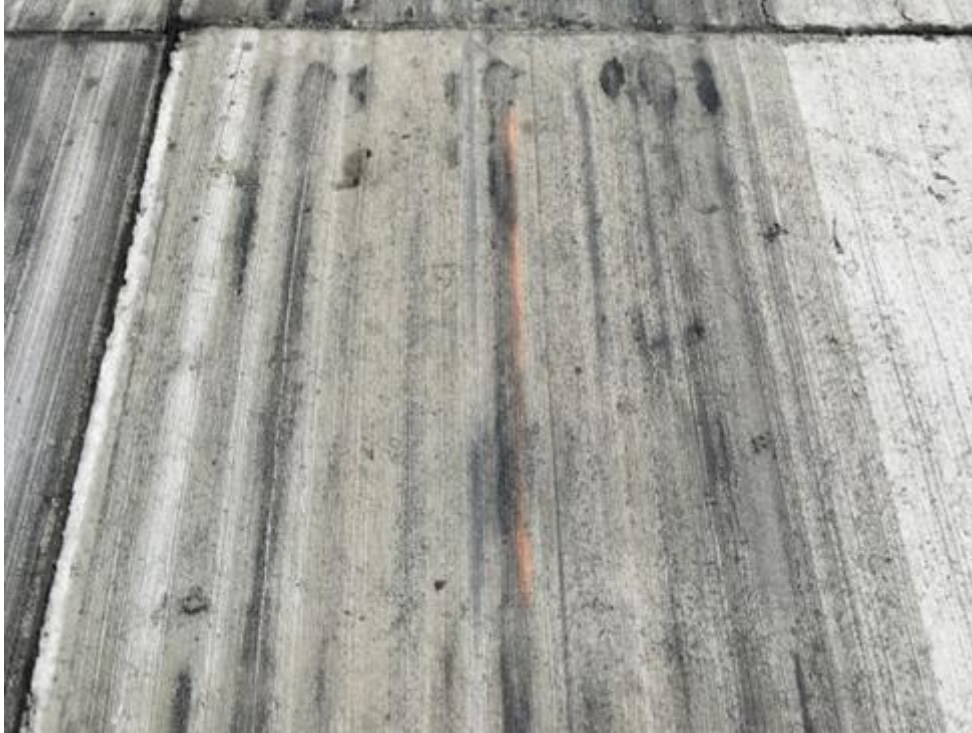
Fig 4.14 Surface of Slab1 ICC-1 after HVS loading.
