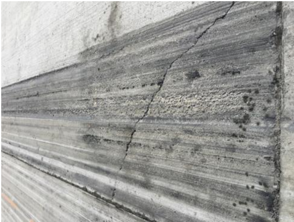
Fig 4.13 Surface of Slab3 ICC-3 after HVS loading.
