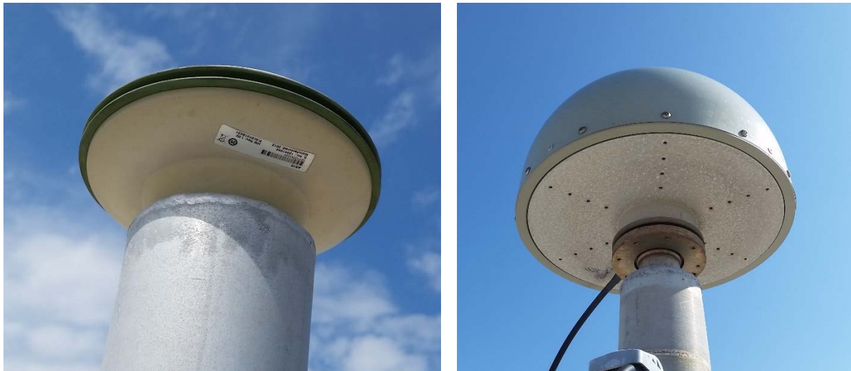
Figure 3-8. GNSS antennae: south end of the main span (left) and center of the main channel span (right).
