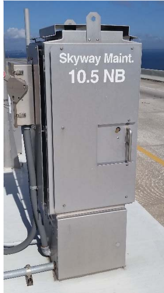
Figure 3-1. An ITS-installed maintenance cabinet located at the center of the main channel span.
