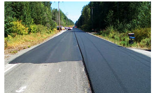
This photo of a repaving project shows the original road surface (lower left), the interlayer (upper left), and the new pavement surface (right).
