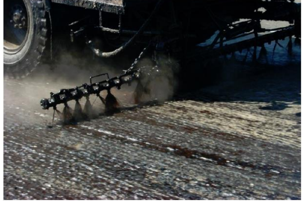
b. Clogged nozzles on SR 500
