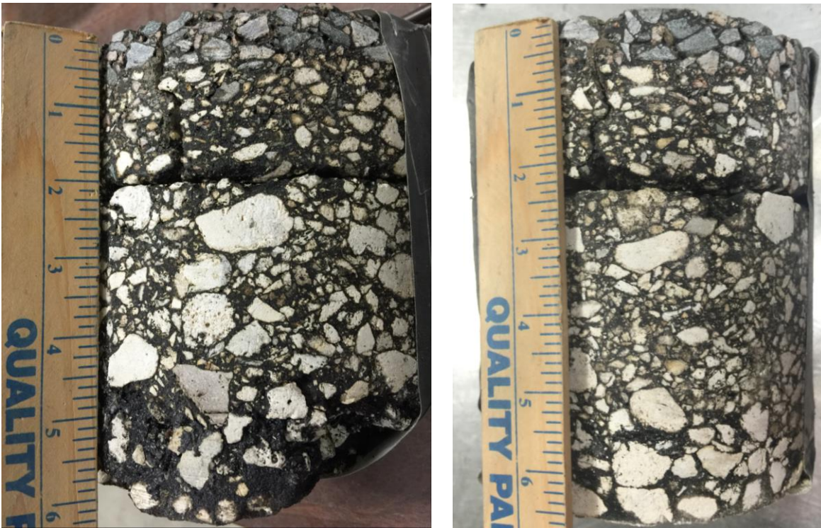
Figure 1-3 Cores exhibiting debonding in combination with near-surface longitudinal cracking (I-10, Duval County). Note: reference measurement in inches.
