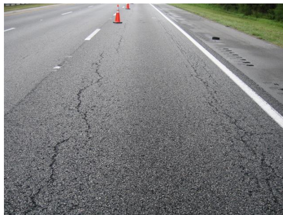
c. Longitudinal cracking in the wheelpath in I-75 (Hamilton County)
