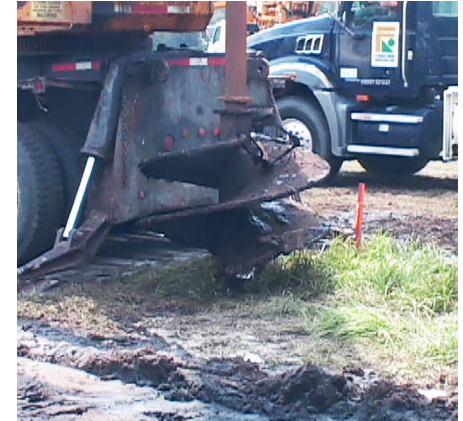
An auger is set in place to drill a hole into which a drilled shaft will be placed.
