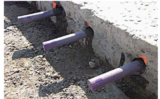
Dowel bars, studied in this project, are set in one slab of pavement waiting for the next one to be poured.
