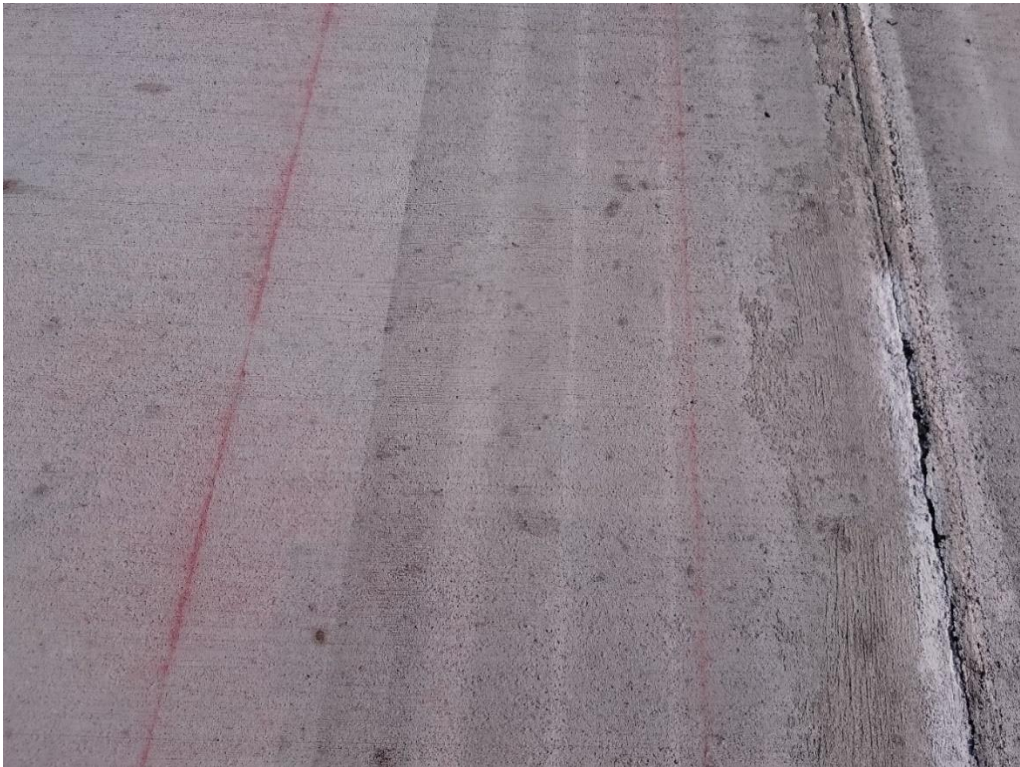
Figure 8-9. Surface of ICC-1 slab after HVS loading
