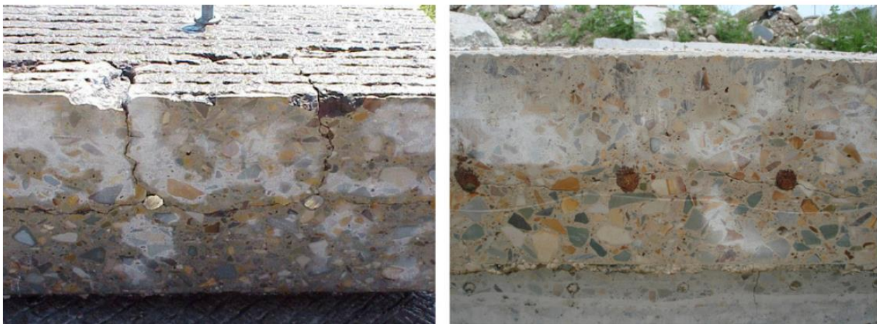
Figure 5-1. Horizontal cracking in CRCP (Choi et al. 2011)
