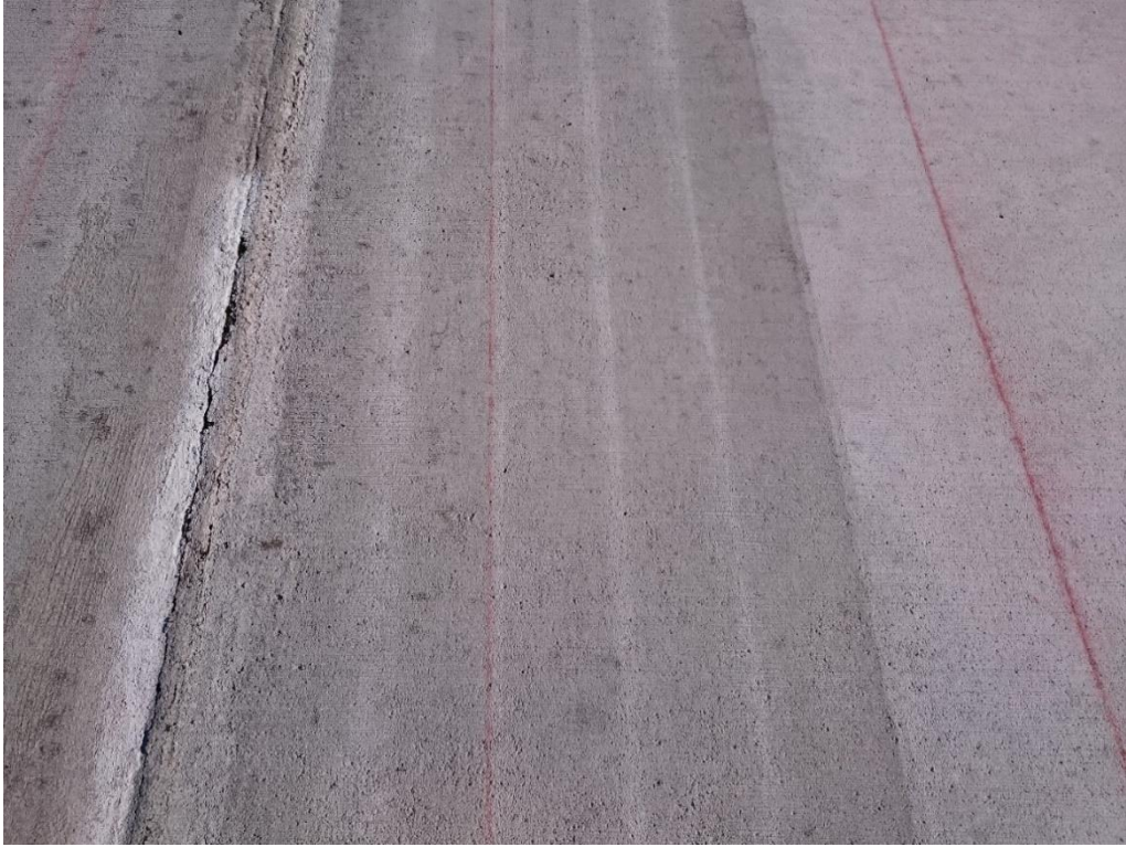
Figure 8-8. Surface of ICC-2 slab after HVS loading
