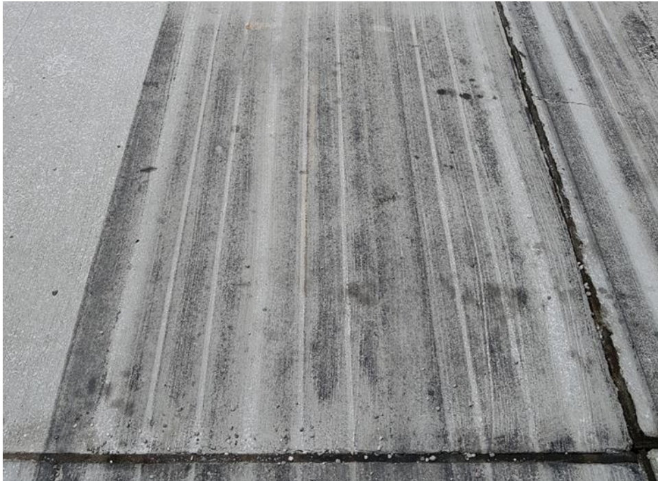
Figure 8-18. Slab 4 after HVS loading
