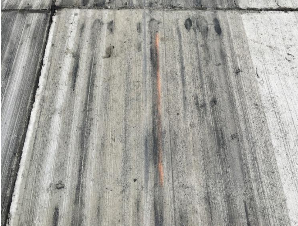
Figure 8-17. Slab 1 after HVS loading
