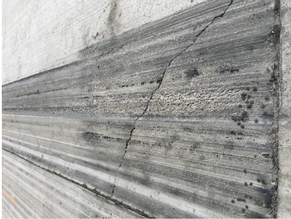
Figure 8-16. Slab 3 after HVS loading
