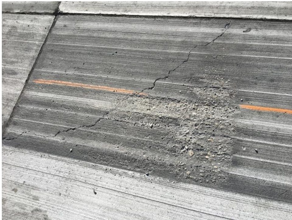
Figure 8-15. Slab 2 after HVS loading
