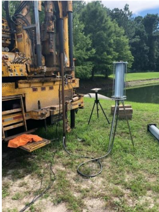
Figure 6.10 The setup of field test in backyard of FDOT using the VAHIP steel probe.
