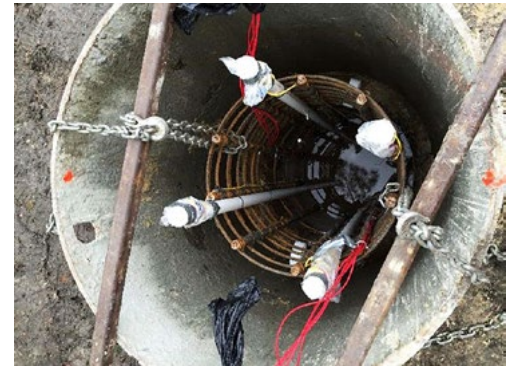
With drilling completed, a rebar reinforcing cage has been placed in this shaft in preparation for concrete.
