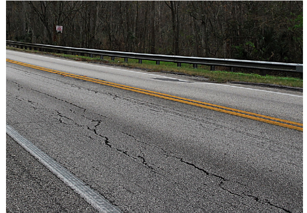
Cracking is an early step in the decay of a road surface. It leads to spalling and potholing, often requiring repeated repair.
