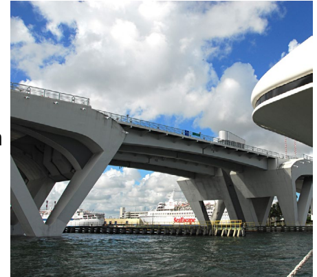
Steel-reinforced concrete is central to many structures like bridges, but it must be protected against water intrusion.
