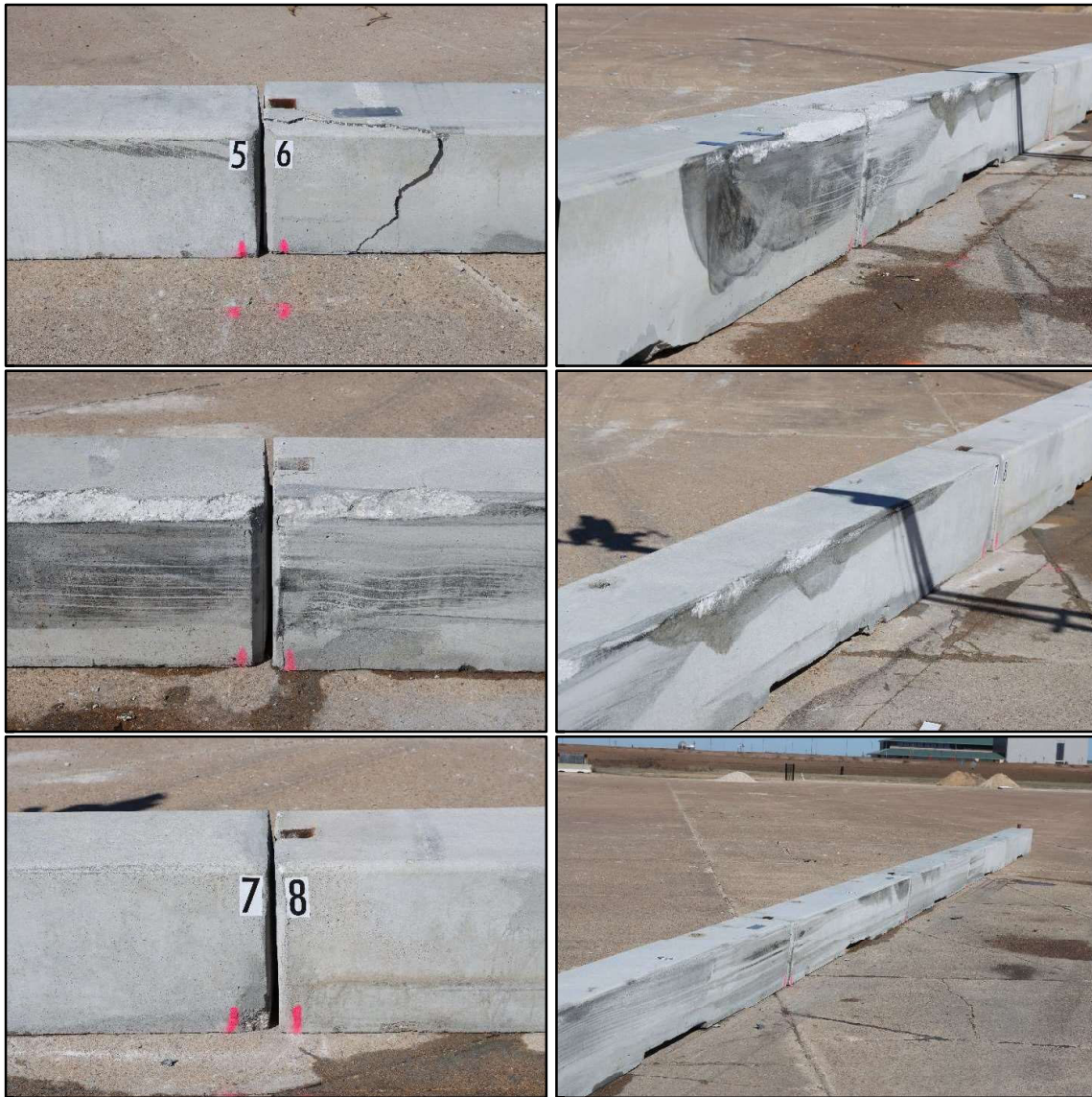
Figure 6.4. Damage to Traffic Side after Test No. 690905-UOF2.
