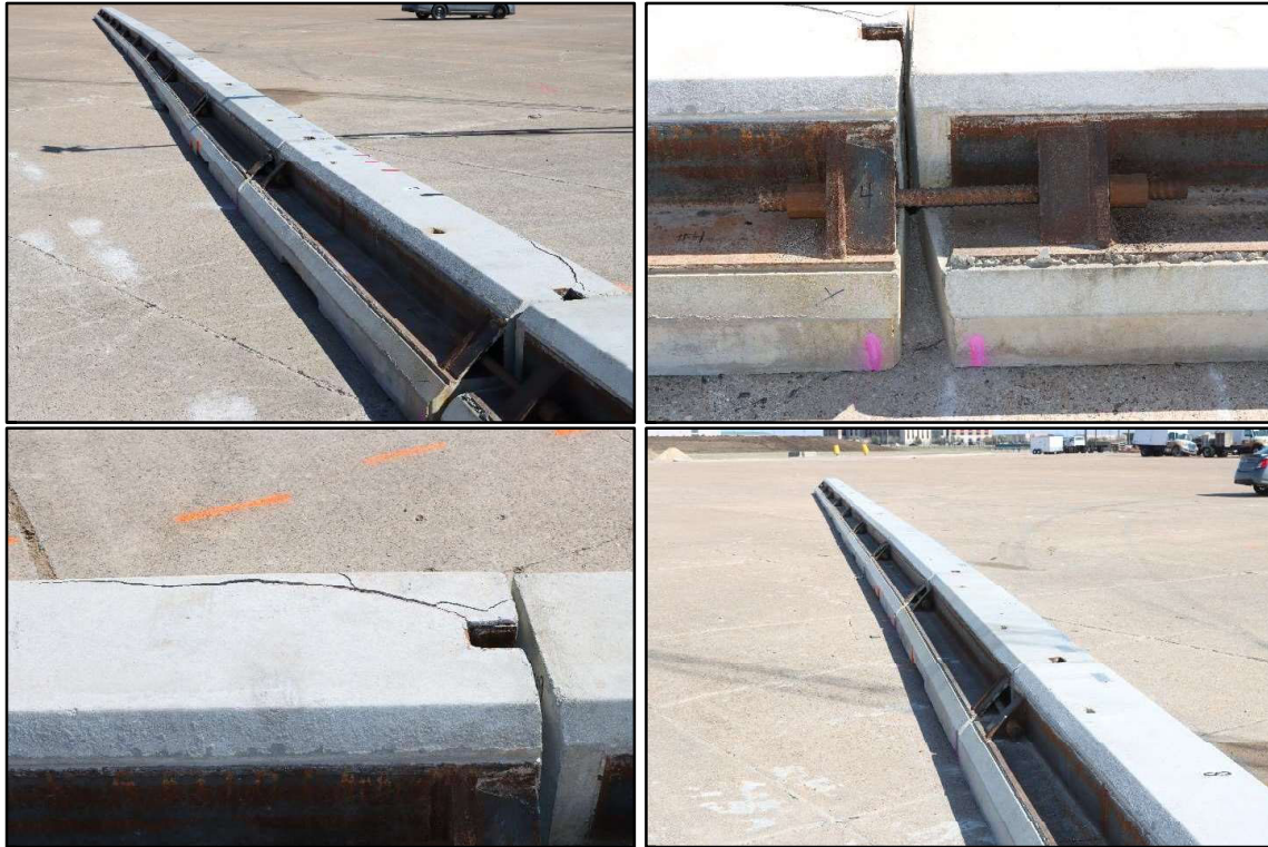
Figure 5.4. Damage to Field Side of Barrier after Test No. 690905-UOF1.
