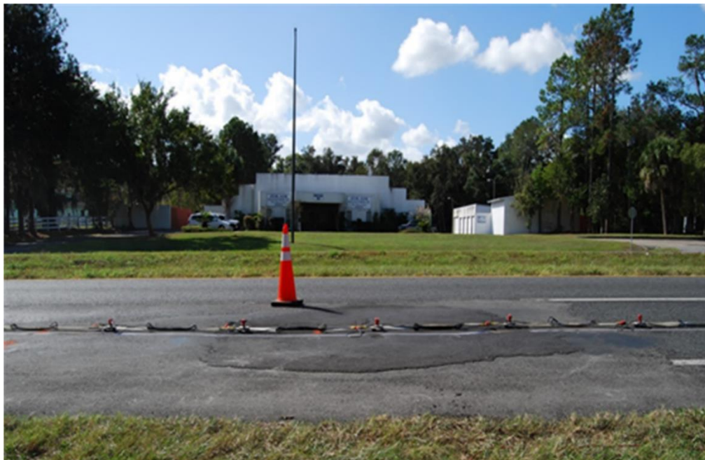
Figure 4.1. US-441 highway test site with a repaired sinkhole (pavement patched area)
