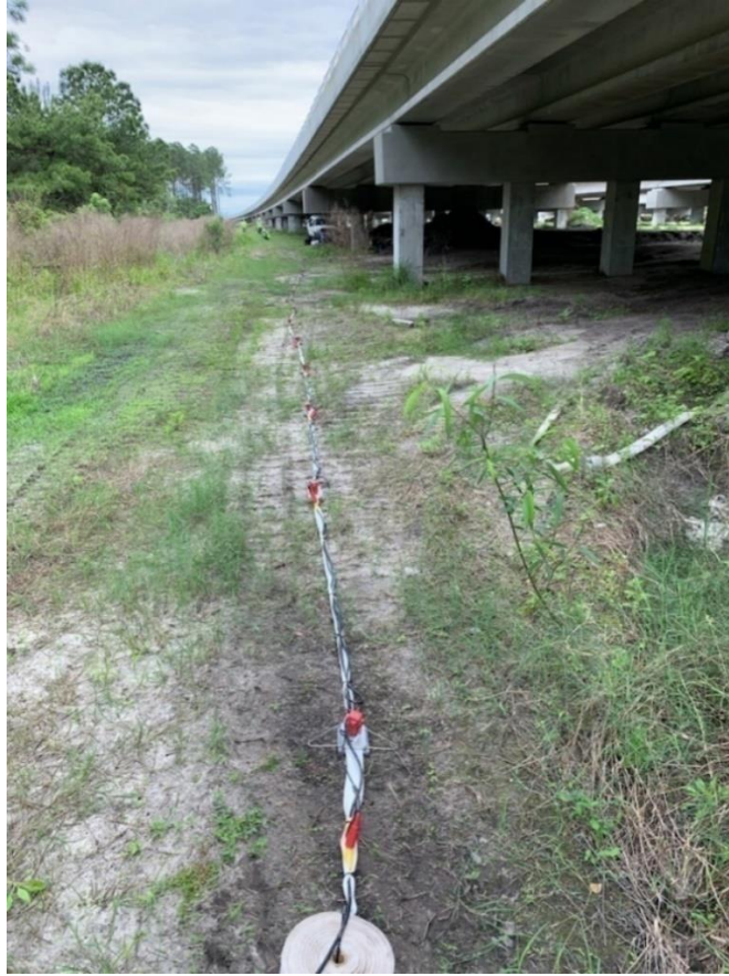
Figure 4.27. Wekiva Parkway, Bridge No. 110110, Bent 3 with problematic soils. A 70-m geophone array was used to record noise data and Bent 3 is at the middle of geophone array at distance of 35 m (117 ft).
