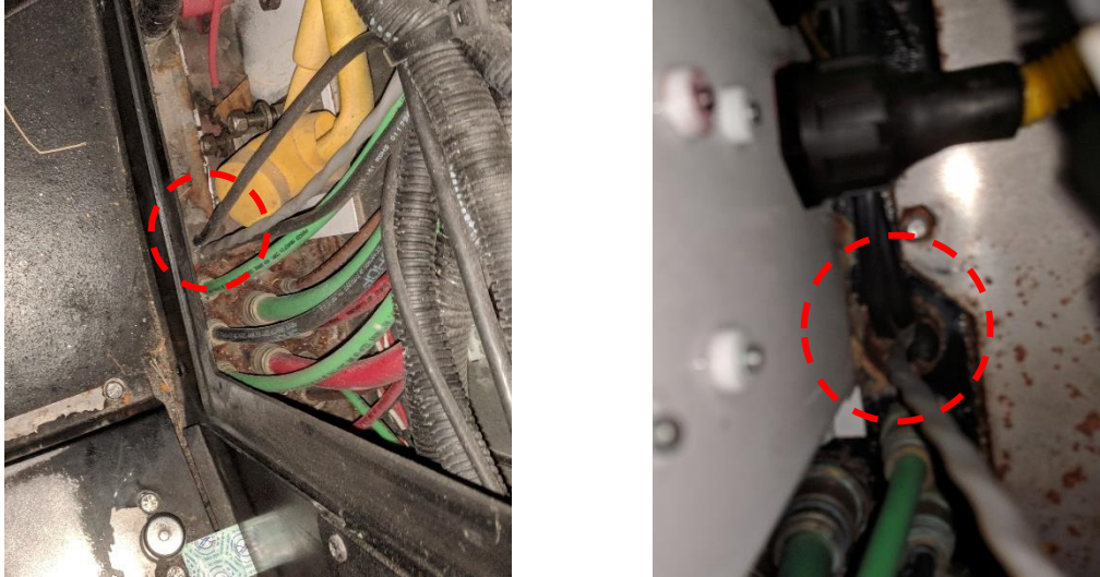
Figure 2-6. (Left) Side panel next to the driver's feet that contains the port to the battery compartment (outlined). (Right) View from the battery compartment of the same port (outlined).
