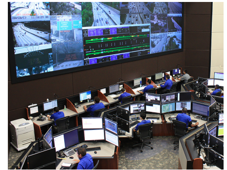
Incidents on Florida Interstates can be managed in real time through regional traffic management centers.
