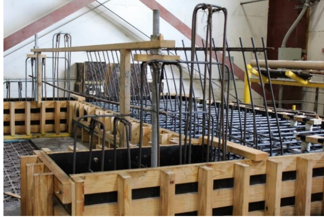
Figure 7-2 Deck-to-rail connection bars and end-support buttress reinforcement positioned inside deck formwork for steel reinforced specimens
