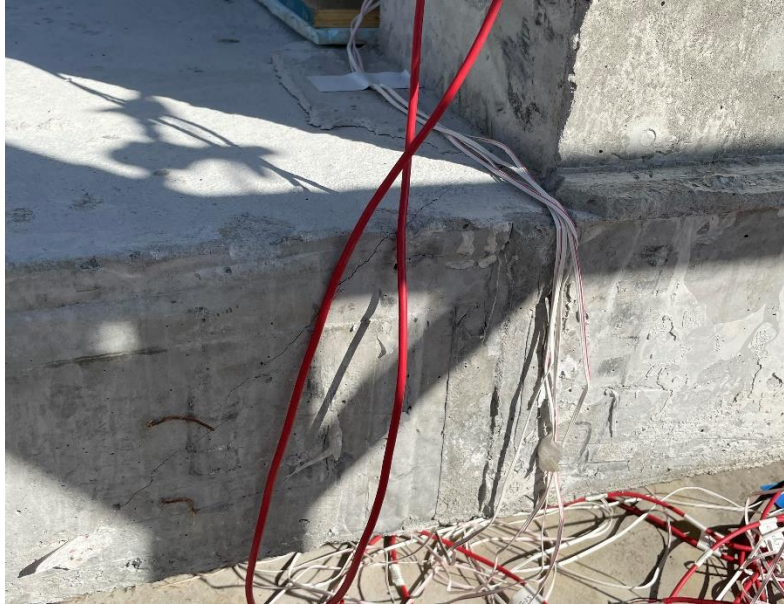
Figure 9-45 Crack in deck with no rail on top (looking towards the back face)
