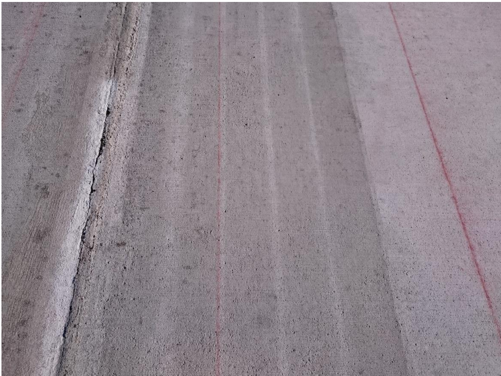
Figure 5-26. Surface of ICC-2 slab after HVS loading.
