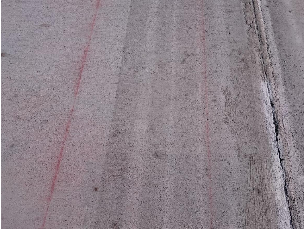
Figure 5-27. Surface of ICC-1 slab after HVS loading.
