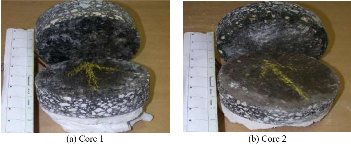
Figure 1-4 Cores taken from areas near Slippage Location 2 (Photos courtesy of FDOT district engineers).
