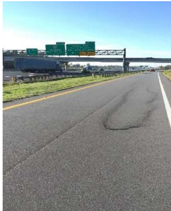
(b) Slippage at Location 2
