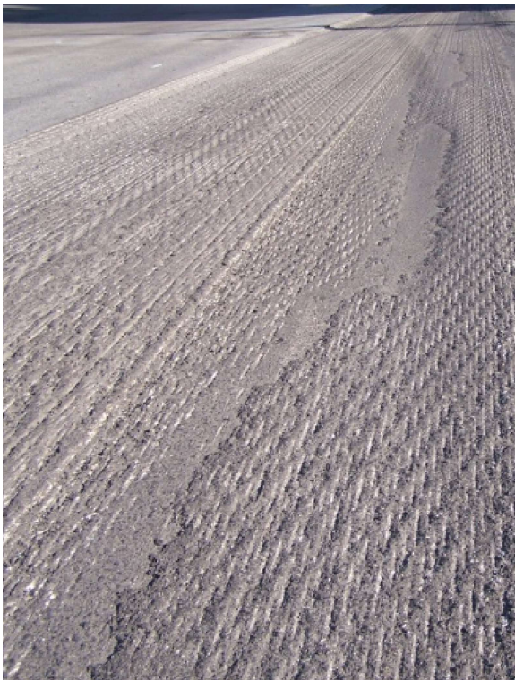
(a) Milled surface of SR 28
