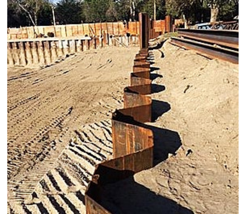
The use of a sheet pile wall to stabilize soil for further construction might be permanent or temporary.
