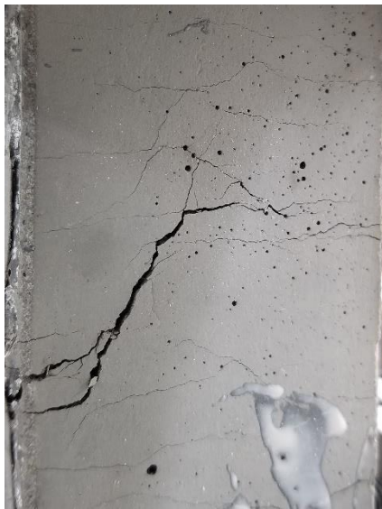
Figure 2-12 Crack localization during tensile loading (Photo credit: Torres)
