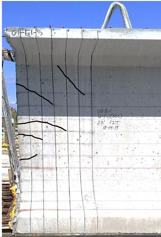
Figure 2-5 End region cracks
