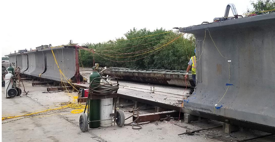
Figure 3-22 Specimens displaced during detensioning
