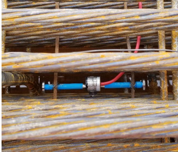
Figure 4-18 Vibrating wire gages used to measure losses
